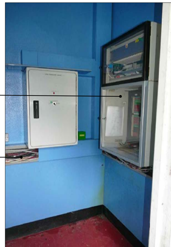
04 015 Ground floor existing electrical room
