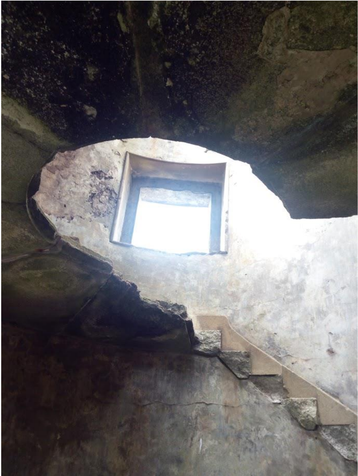
Fig. 7 – View of interior of lighthouse tower and ruined cantilevered staircase.
