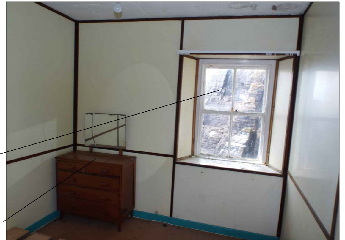
02 036 Image showing a room located on the ground floor of the lower lighthouse
