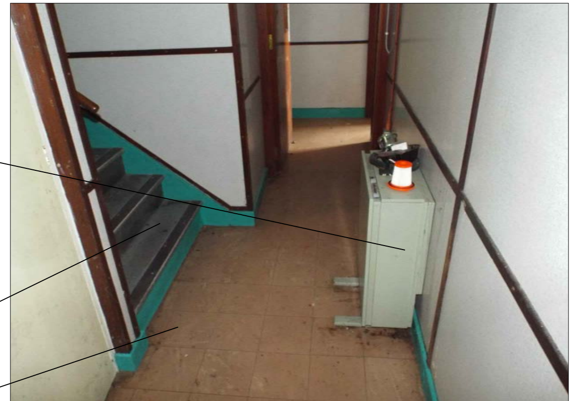
04 036 Image showing the hallway on the ground floor of the lower lighthouse
