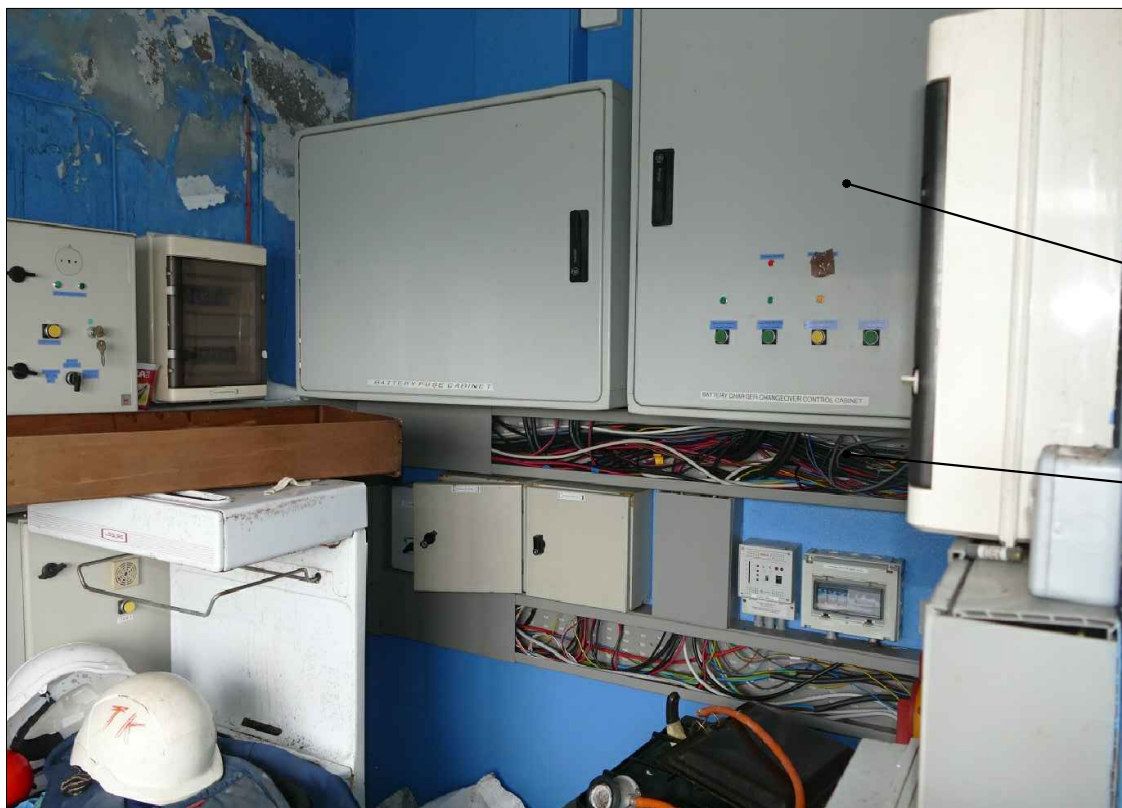
03 015 Ground floor existing electrical room
