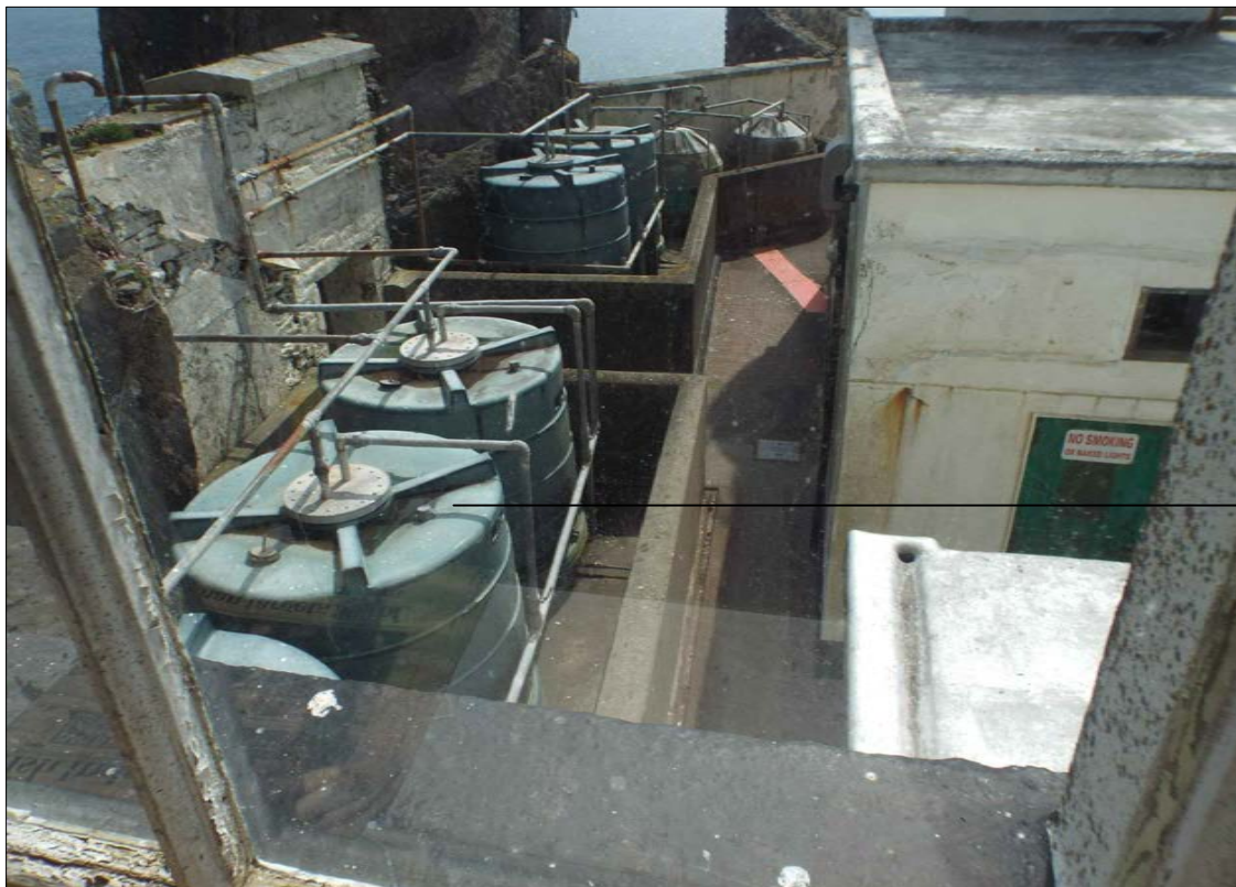
02 Image showing the tanks on the ground floor level of the lower lighthouse
