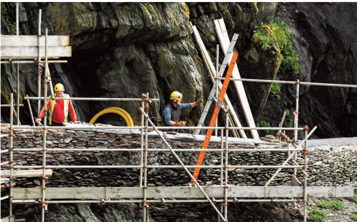
Pl. 18 Relaying Valentia slate capstones on the sea wall north-east of the Lower Lighthouse complex.
