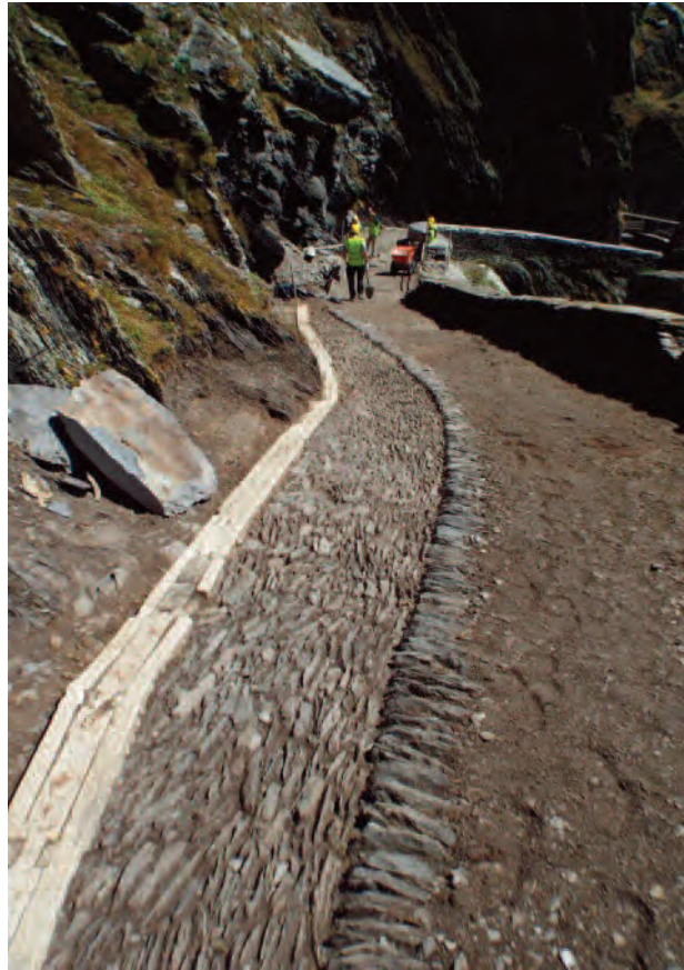
Pl. 31 The Upper Lighthouse Road, after excavation, showing the original road surface, drains and an electrical conduit inserted in the early twentieth century.
