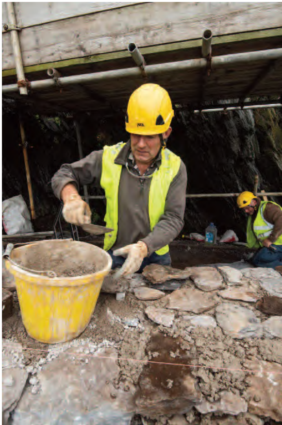
Pl. 19 An OPW mason laying the base for new capstones on the sea wall, Upper Lighthouse Road.
