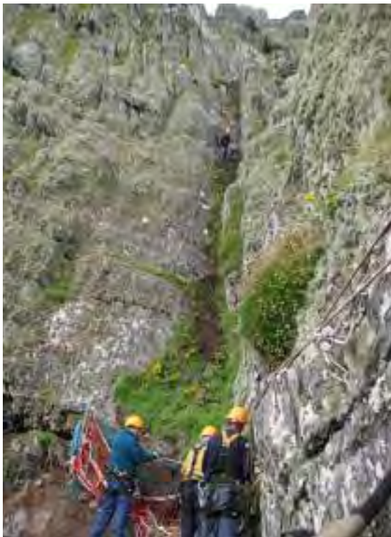
[Left] Ill. 2.290—Looking up the gully from the end of the northern traverse at the start of excavations (A.R. Hayden).
