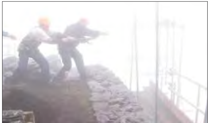
Ill. 2.531—Even when the winch broke down, the OPW crew still managed to haul, by hand, a substantial quantity of stone up to the oratory terrace from the ledges below (A.R. Hayden).
