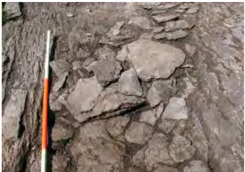
Ill. 2.195—Detail of slipped step riser; visible at the left of the preceding photograph (A.R. Hayden).
