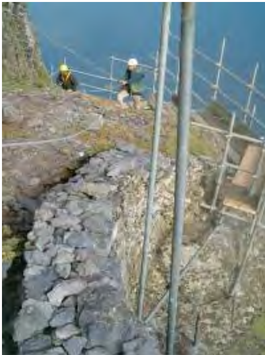
[Right] Ill. 2.365—Only the basal stones of the wall survived at the south-eastern end of the terrace. Note the loose and slipped stones ready to fall (A.R. Hayden).
