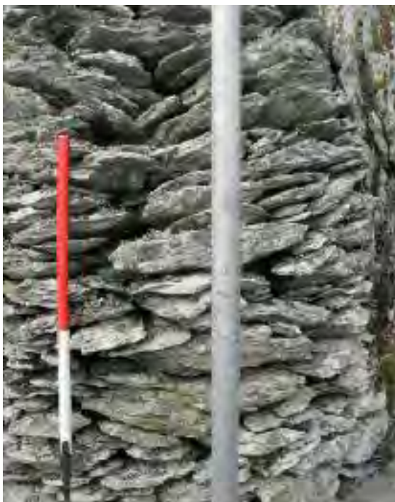
[Left] Ill. 2.503—Vertical crack in the wall south of the south-western corner (A.R. Hayden).
