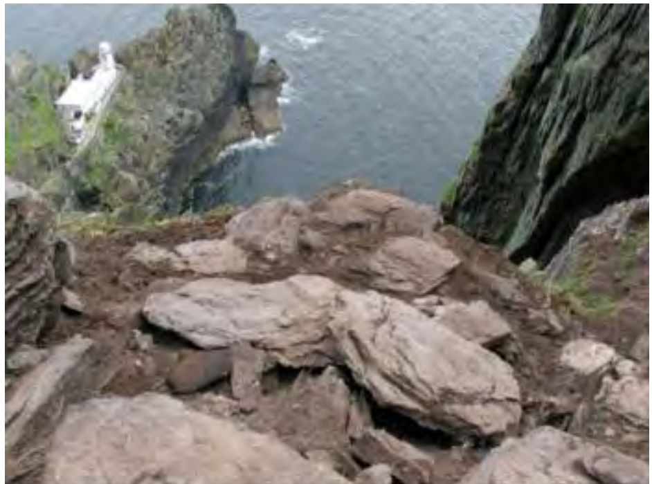
III. 2.248—Looking down on the first section during excavation. Collapsed paving slabs can be seen in the foreground, and part of the surviving traverse wall at the back (A.R. Hayden).
