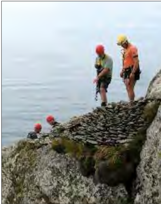
[Right] Ill. 2.475—The highly collapsed and unstable centre of the western wall of the terrace (A.R. Hayden).
