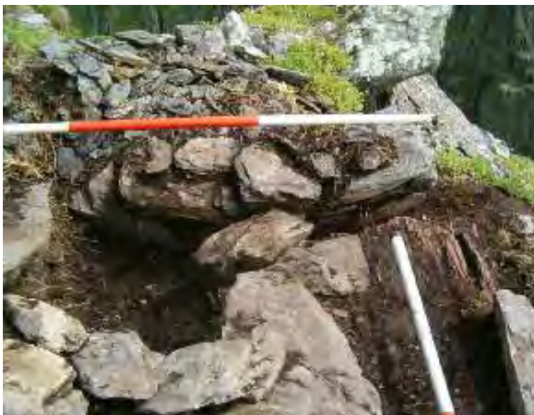
Ill. 2.410—The southern end of the inner face of the east wall. Note how it has twisted and moved (A.R. Hayden).
