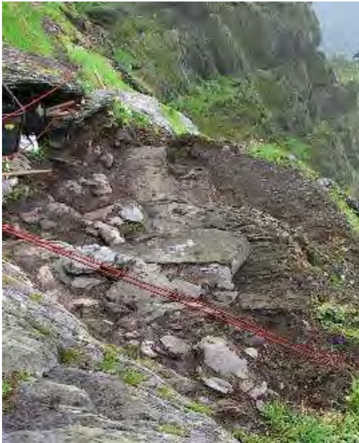
Ill. 2.331— Remnants of masonry steps between the stepped ledge and the base of the cliff beneath the Needle's Eye (A.R. Hayden).
