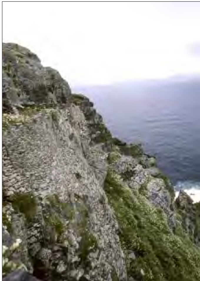
Ill. 2.2—The small oratory terrace retaining wall, looking north, before works (A. Lynch).
