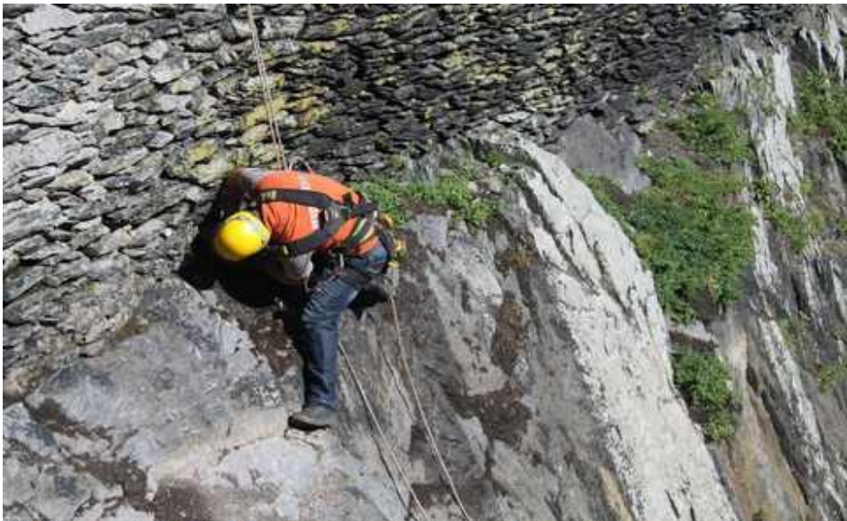
Working on the repair of the retaining wall after the removal of the cementitious repair.
