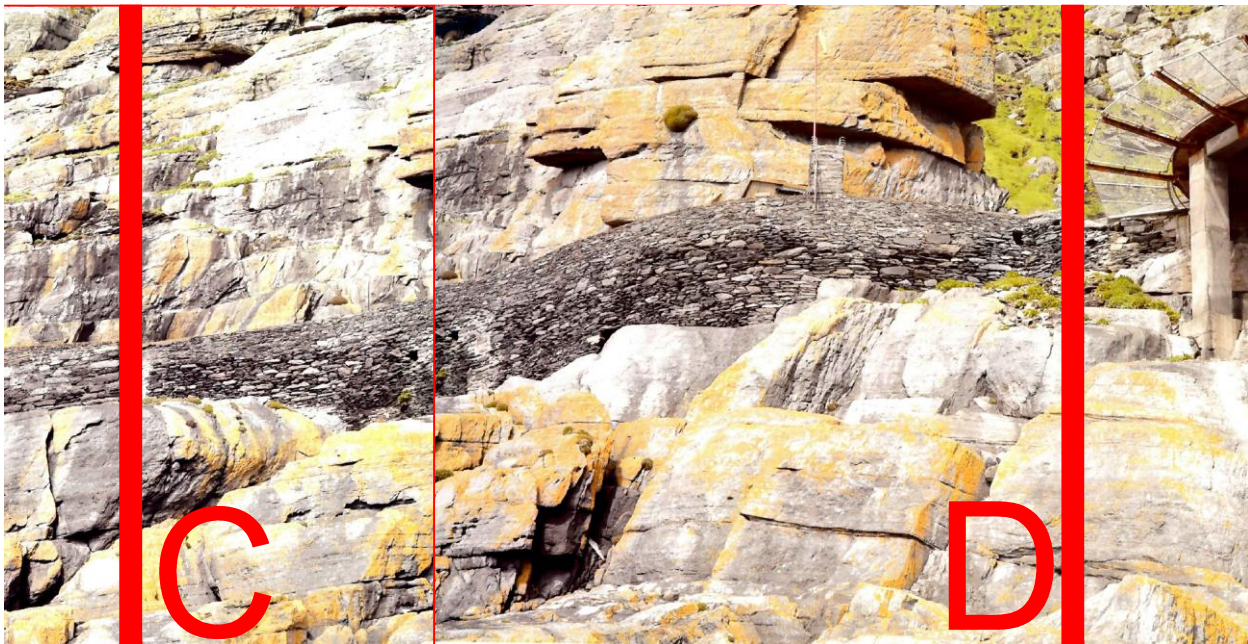
Retaining wall C-D. See plan, as this actual stretch runs up to the point E to the left. This section of walling (E-D) was completed in 2014.
