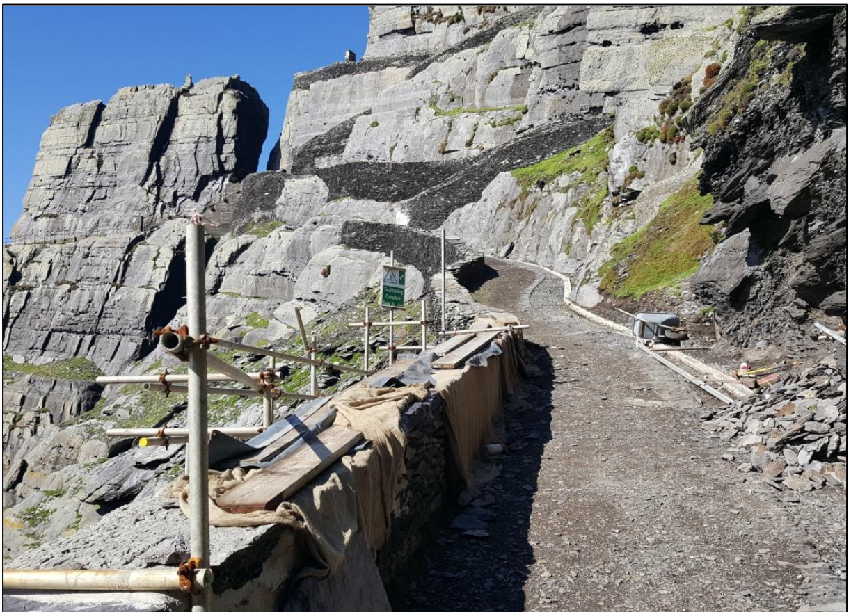
Figure 5. Typical road surface along Upper Lighthouse Road following removal of surface vegetation and infilling
