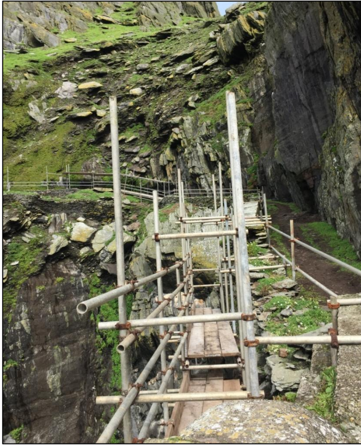
Figure 2: Typical scaffolding set-up along breached section of seawall and roadway
