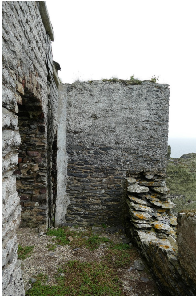
Figure 5 - Existing debris in Upper Lighthouse
