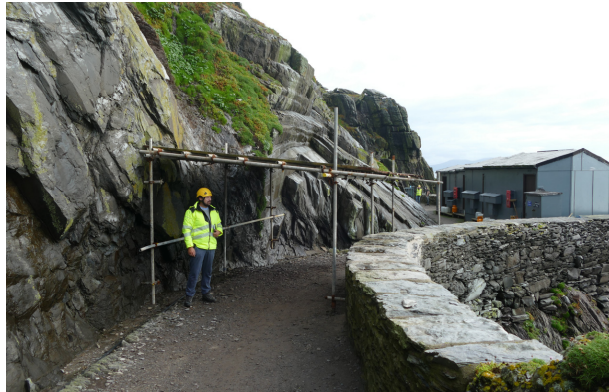
Fig. 28. – Temporary crash deck location A near site huts and installed following rock-fall.
