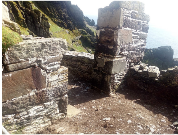
Fig. 11. – View of Outer Gate to Upper Lighthouse. It is currently in a precarious condition and will require repair in 2021 to prevent further deterioration.
