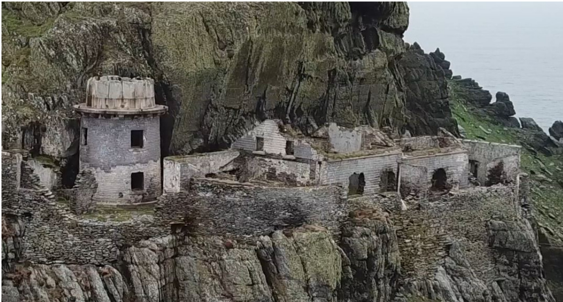
Fig. 30. – Proposed repairs to Upper Lighthouse sea wall and removal of debris from buildings in 2021 Season.
