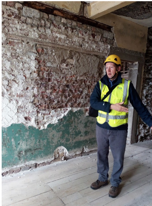
Fig. 23 - OPW Senior Conservation Architect Fergus McCormick inspecting repair works to the Lower Lighthouse.
