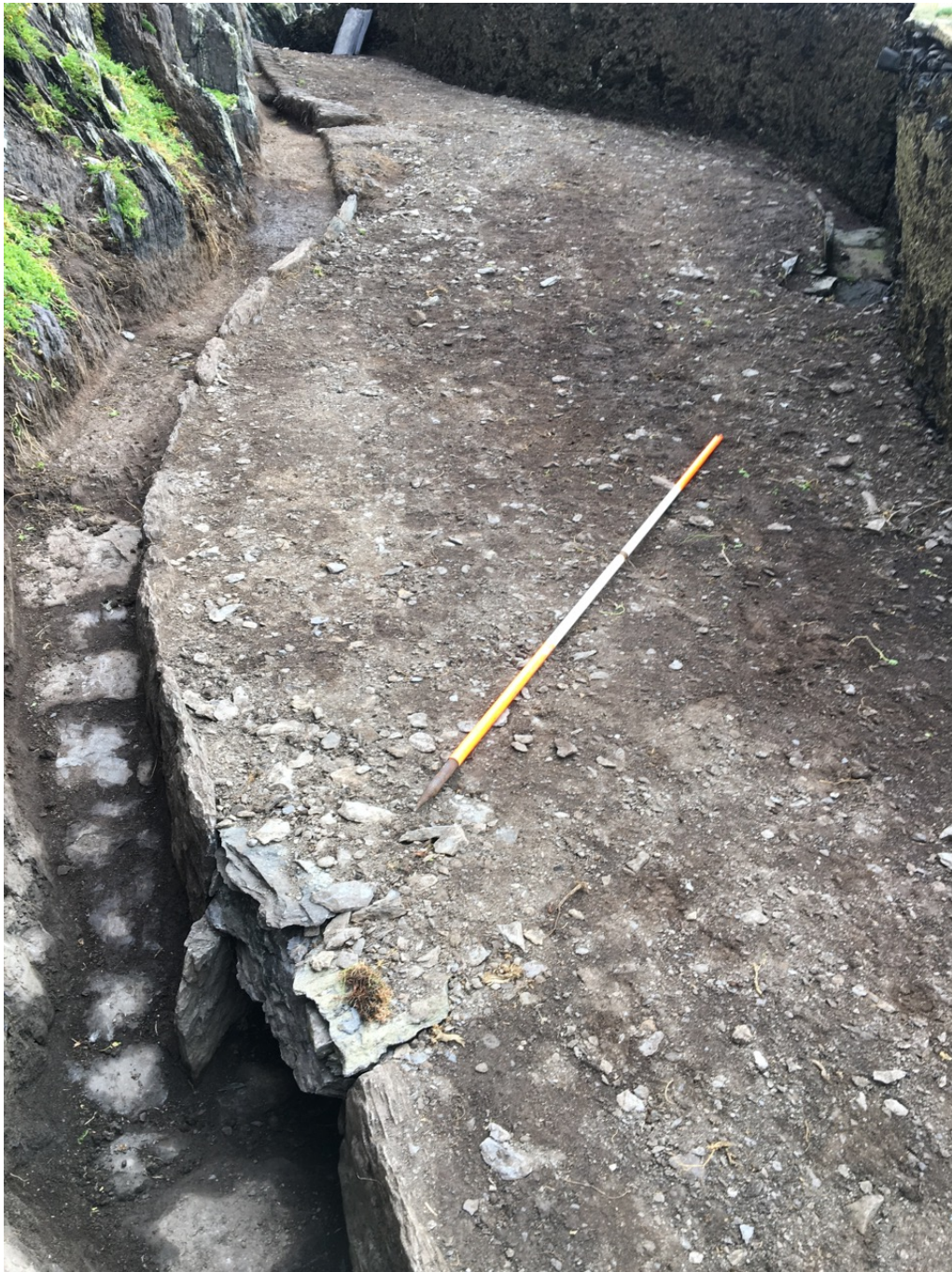
Photograph 17, section E3 looking east. Opening of subsurface drain into lateral drain at left and surface drain at right (see photograph 18). Replaced road edging in foreground with rock cut lateral drain and original road edging in background.
