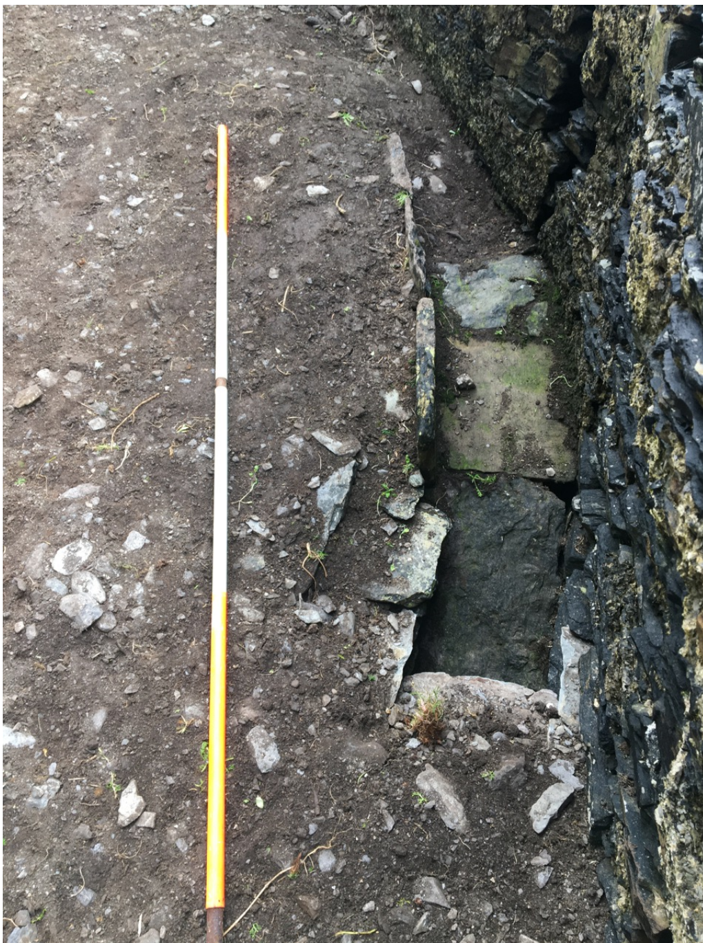
Photograph 18, section E3 looking east. Surface drain inside parapet wall. Note large crack in parapet wall.
