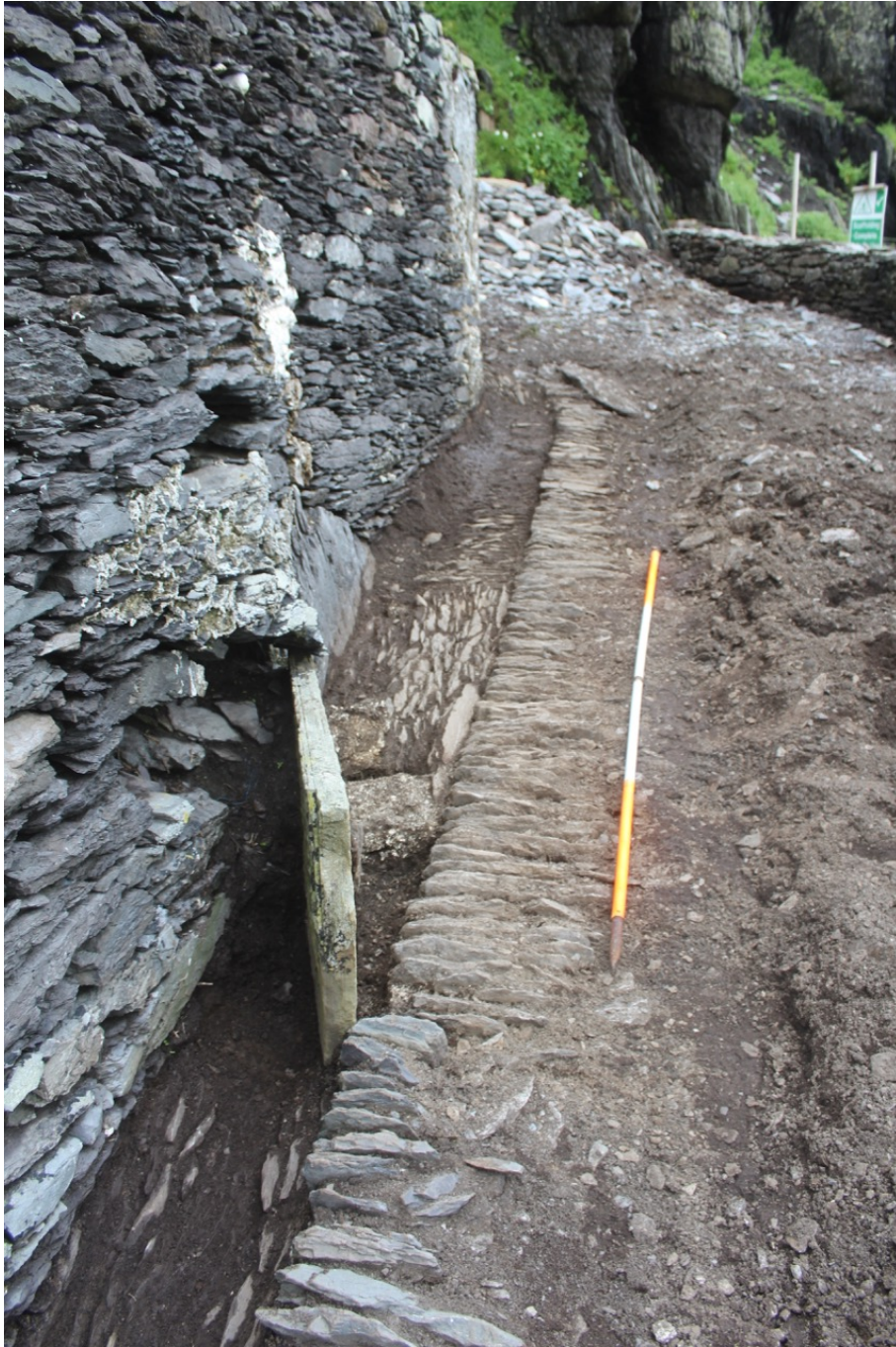
Photograph 5, section E1 looking east. Replaced road. Edging at front, partly collapsed base of parapet wall and inserted vertical stone with original road edging and intact lateral drain behind, note stones in base of lateral drain laid at right angles to its line at back.
