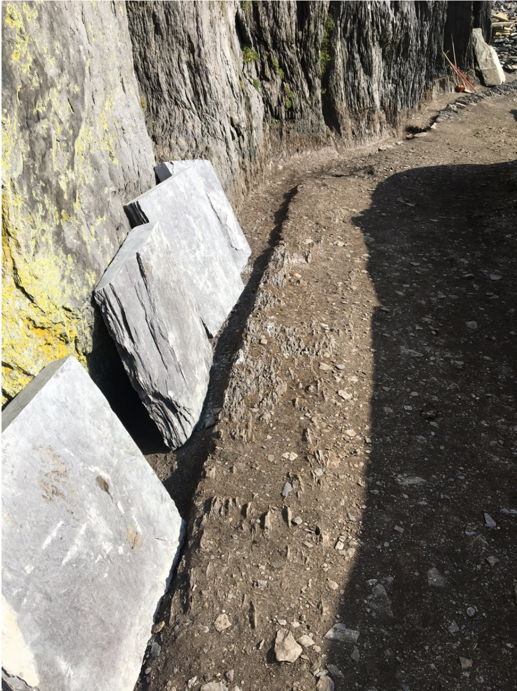
Photograph 24, section E4 looking east. Exposed rock at road surface and rick cut lateral drain.
