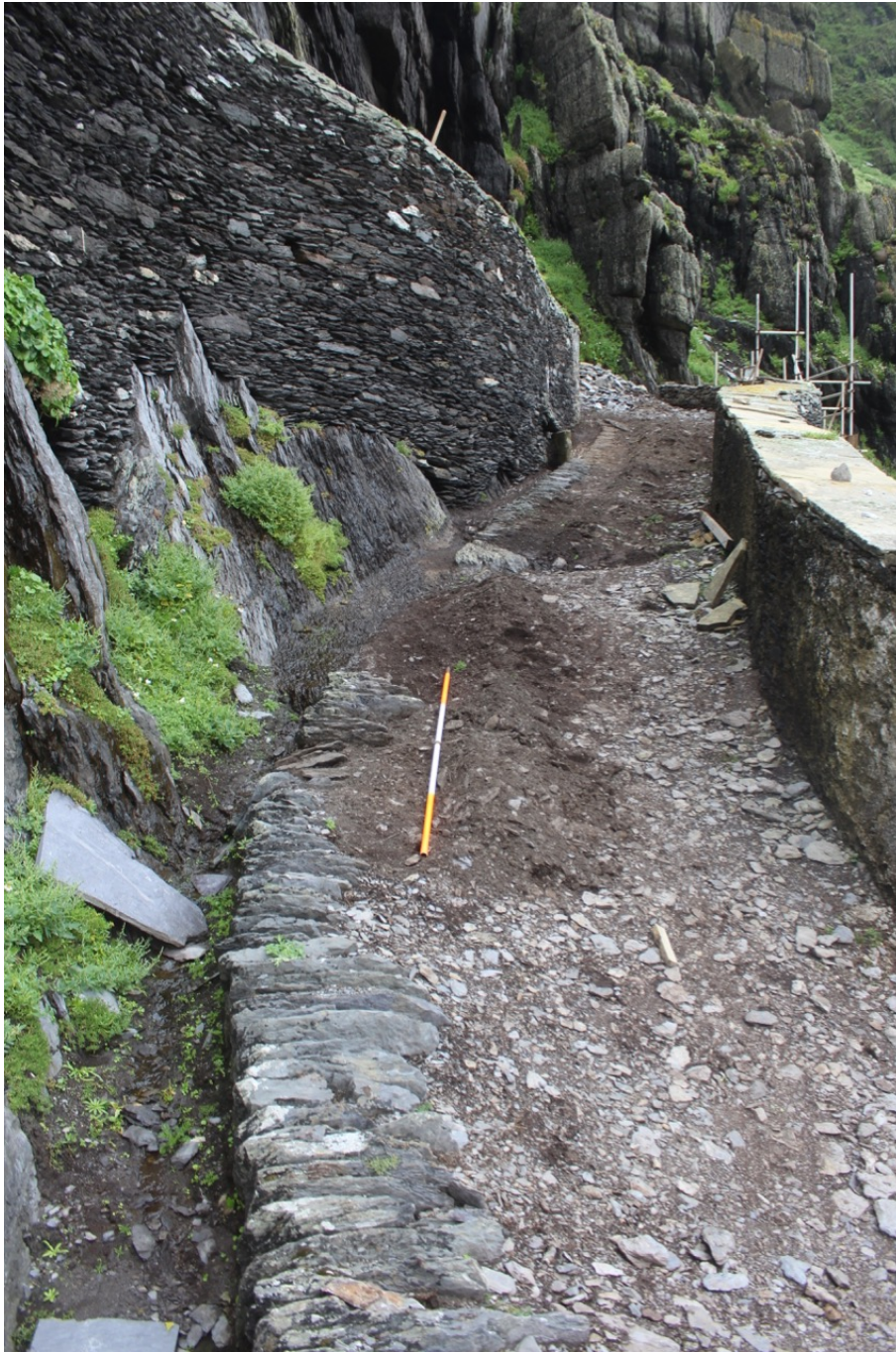
Photograph 1. Section E, looking east. Intact road edging with damaged section by ranging rod and damaged lateral drain base at left. Surviving surface of roadway below original level.
