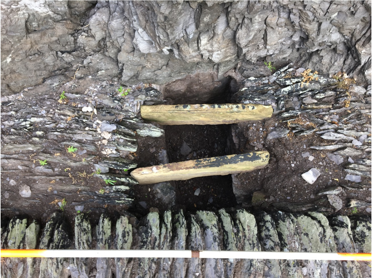
Photograph 8, section E2 looking north. Stone shore (several stones missing) in lateral drain, overlying subsurface drain.
