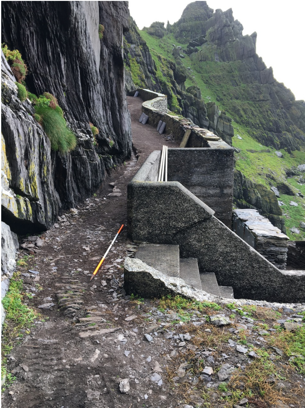
Photograph 15, section E3 looking east. Short length of intact road edging in foreground. Mass concrete walls with road edging replaced by vertically set flags at back left.
