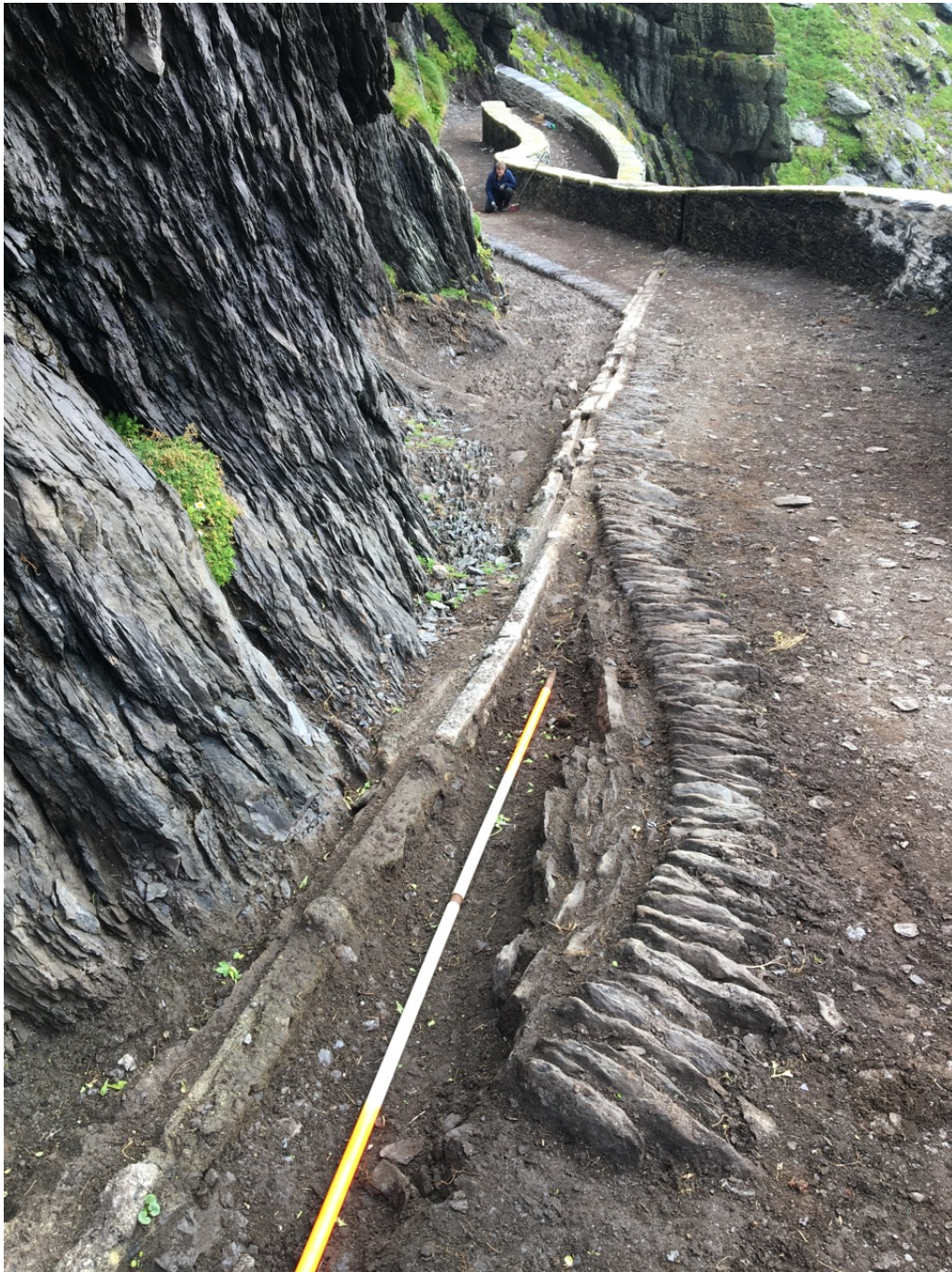
Photograph 11, section E2 looking east. Cable channel cut through base of lateral drain, gaps in base of lateral drain and road edging removed in foreground.
