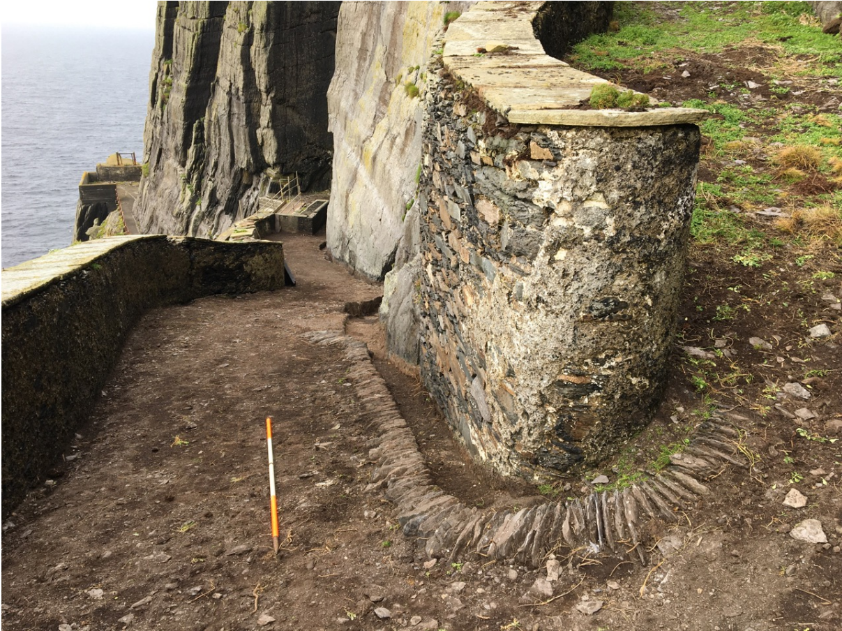
Photograph 21, section E3 looking west. Road edging and lateral drain curving around parapet wall, road surface slightly below original level.
