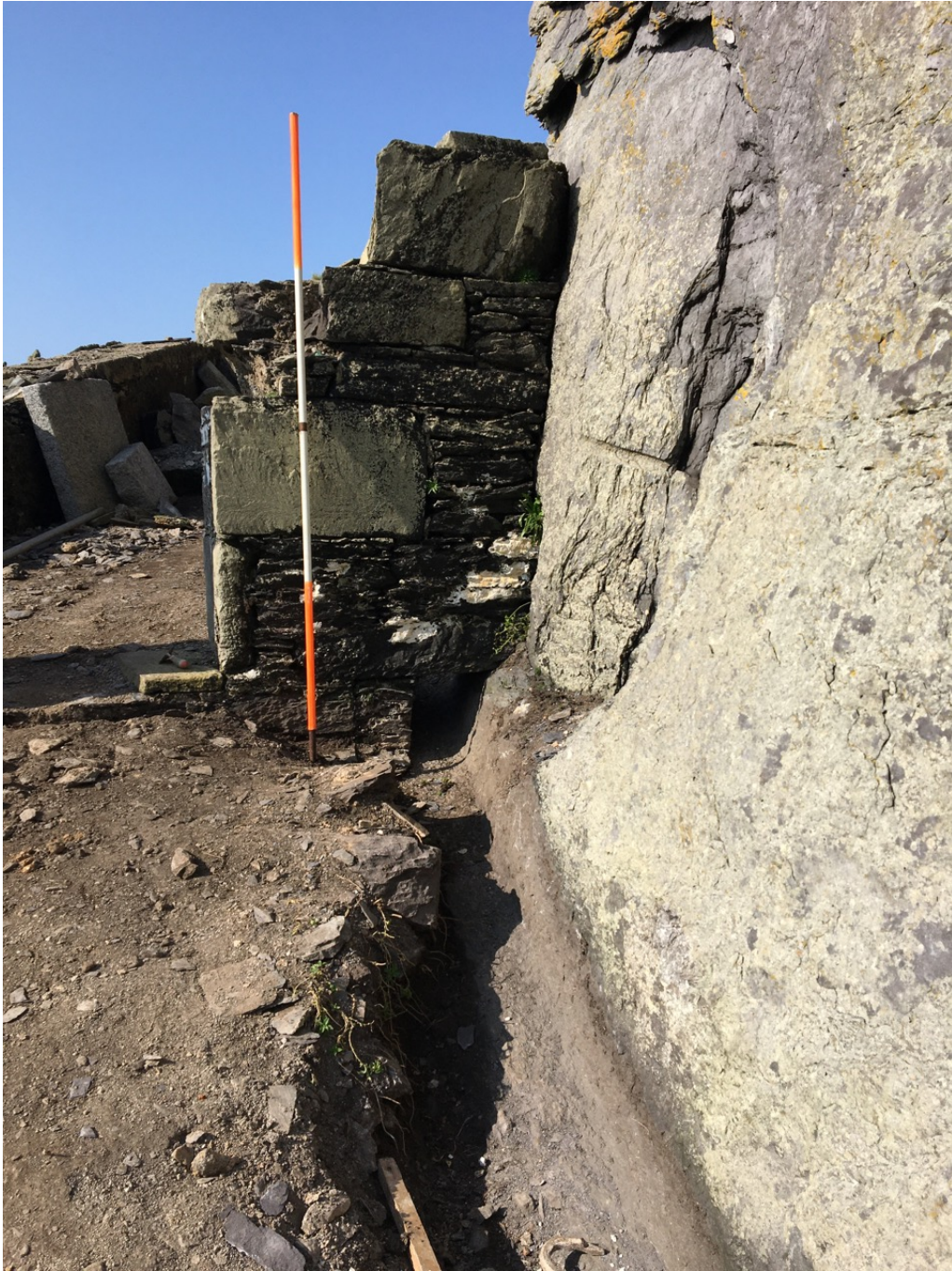
Photograph 24, section E4 looking west. Rock cut lateral drain narrowing and extending beneath gate of Upper Lighthouse.
