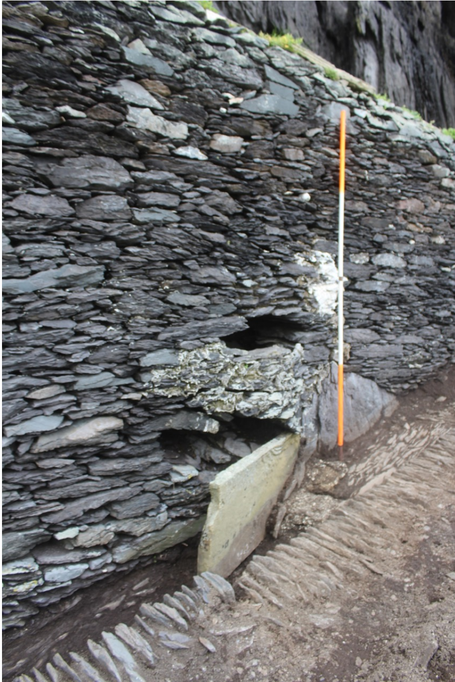
Photograph 4, section E1 looking north. Partly collapsed base of parapet wall with drain exit and inserted vertical stone secured with cementitious mortar. Rebuilt road edging at left, original at right.
