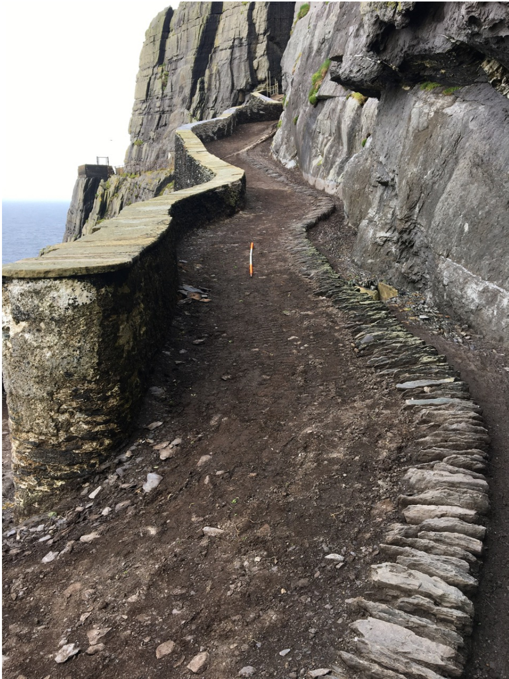
Photograph 7, section E2 looking west. Well preserved road edging and lateral drain. Road surface below original level. Shore (see photograph 8) in lateral drain at right.
