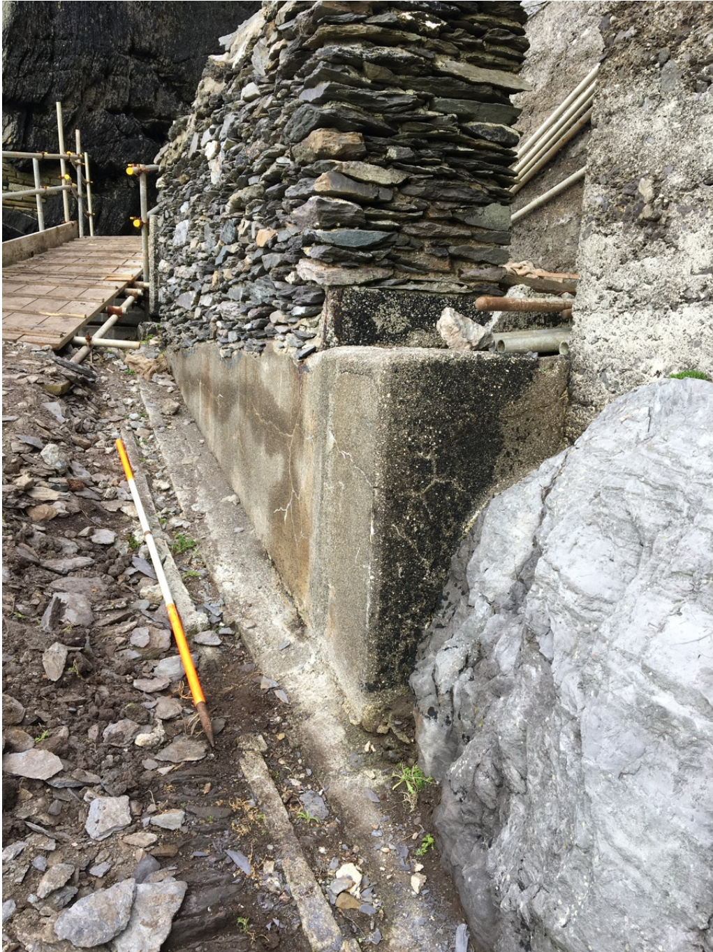
Photograph 14, section E2 looking west. Cable channel at base of mass concrete wall topped by modern bird-nesting wall.
