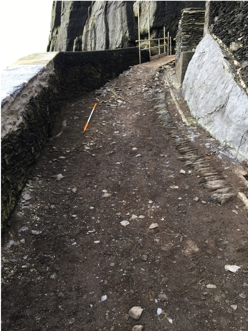
Photograph 12, section E2 looking west. Removed and intact road edging with lateral drain cut by cable channel at right and surface drain (to left of ranging rod). Mass concrete wall and modern bird-nesting wall in background.
