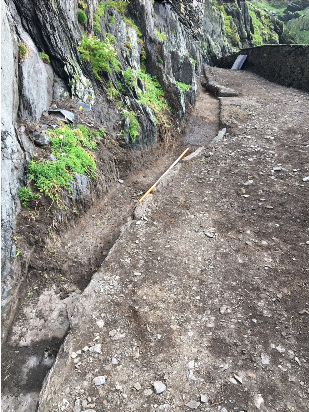
Photograph 19, section E3 looking east. Original road edging replaced with vertically set flags, rock cut base of lateral drain, original road edging in background.
