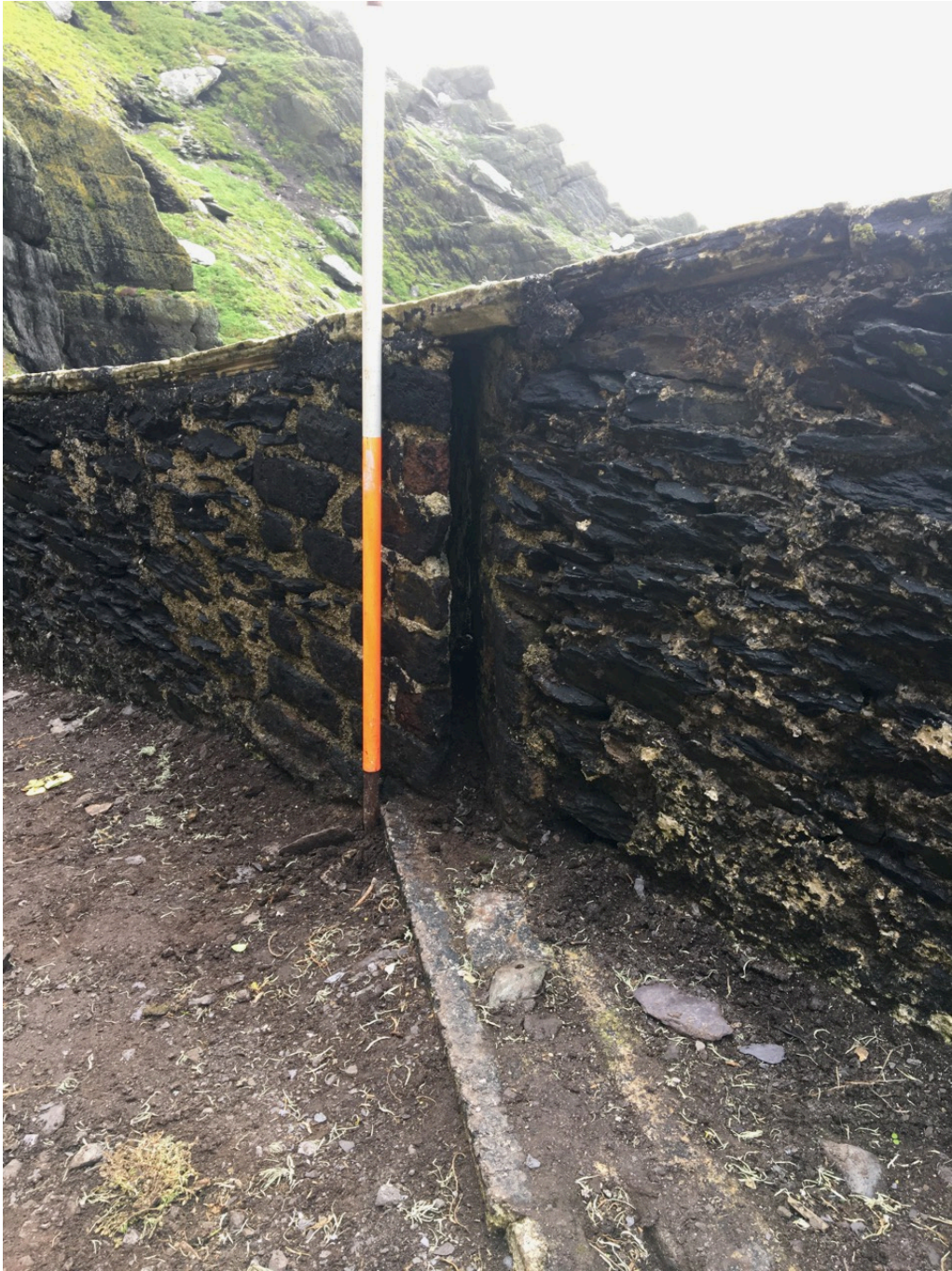
Photograph 10, section E2 looking southeast. Slot in parapet wall for cable with cable channel in foreground.
