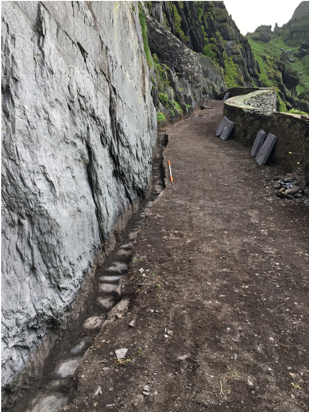
Photograph 16, section E3 looking east. Original road edging replaced by vertically set flags and flagstone base of lateral drain.
