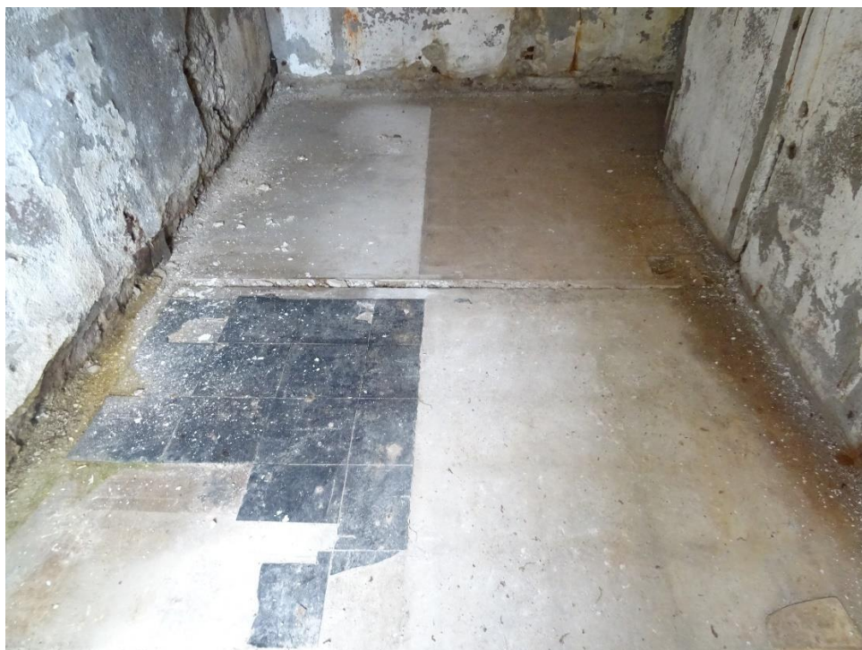
Figure 4. Poured concrete floor at ground floor level with a portion of tiles remaining in place (Carrig, 2020).
