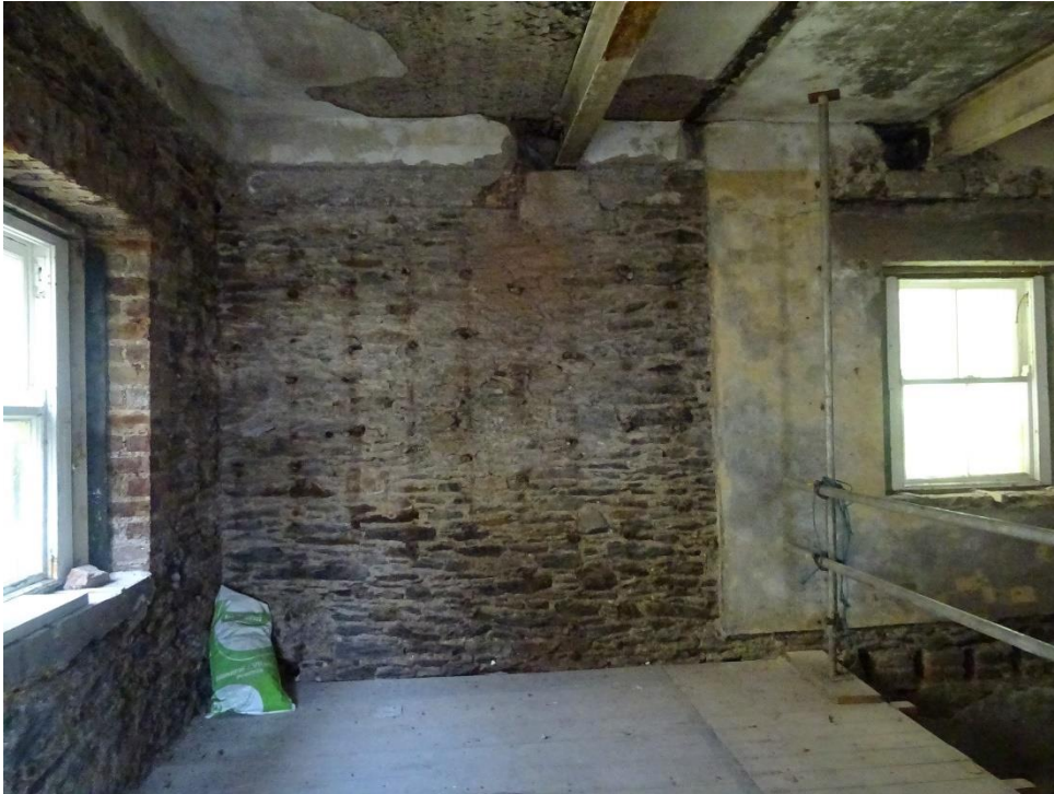
Figure 5. Random rubble external walls with brick window surrounds on the first floor (Carrig, 2020).
