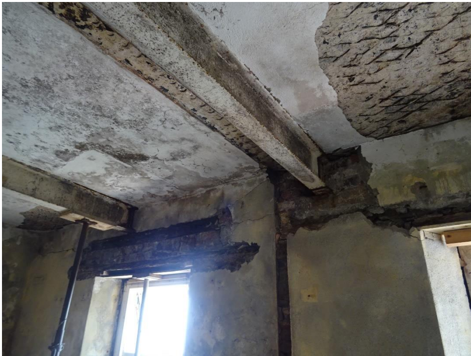
Figure 9. Underside of the reinforced concrete roof. Both the reinforcing mesh and steel I-beam supports are showing signs of corrosion (Carrig, 2020).
