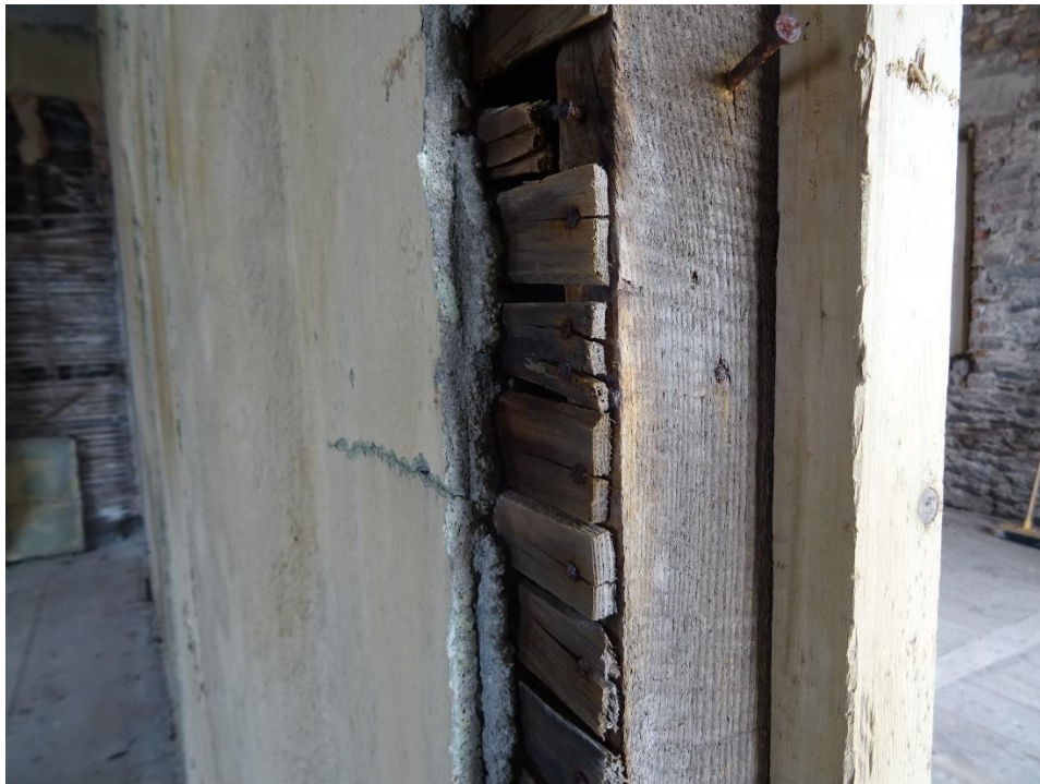
Figure 6. Lath and lime plaster in-situ on an internal wall on the first floor (Carrig, 2020).
