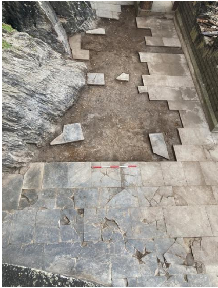
Fig.101. Cracked paving south of the lighthouse (11).
