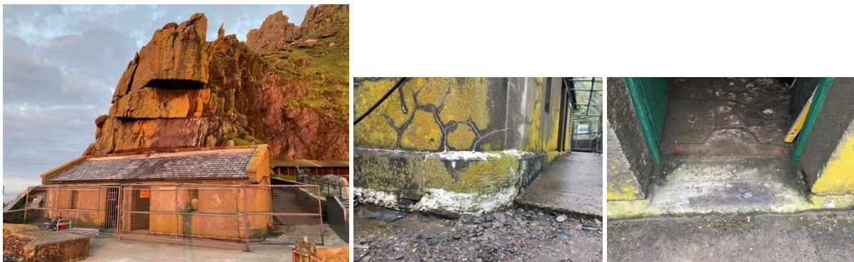
Fig. 174. The shed by the helipad and details of its plinth & door cills.
