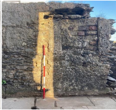
Fig.124. East wall of Shed (21) with wall scar (sunlit) & blocked window.
