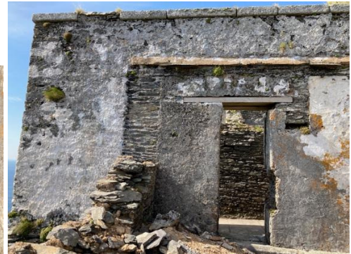
Fig.128. Scar of south wall of Shed (23).
