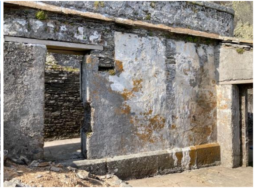
Fig.125. Wall scars and roof line of Shed (21) on Outer face of wall (5) around yard (9).
