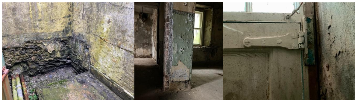
Fig.171. (l. to r.). The toilet of the Lower Station with its sandstone skirting; possibly the last surviving original sandstone skirting in the houses of the Lower Station, and a hinge on the original front door in the Lower Station Houses, which is identical to that found in the Upper Station (see find. No 55, fig. 157).
