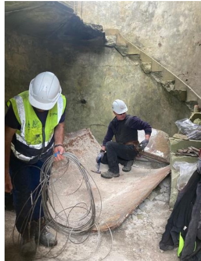
Fig.90. Preparing to move the collapsed back of the lantern.
