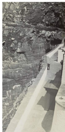
Fig. 170. The slate weathering on the Lower Station.
