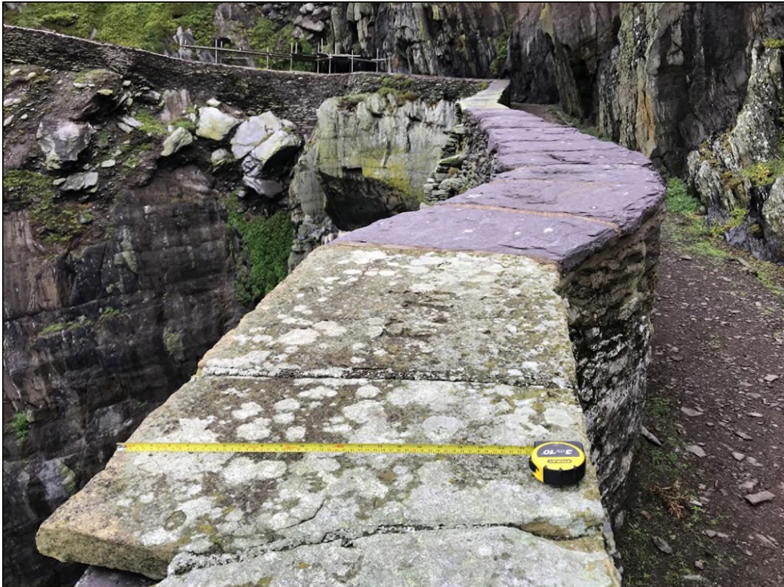
Photograph 9: Lighthouse Road Lower Section. Yorkshire Flagstone Cap in Foreground, "New" Valentia Slate Caps in Background.
