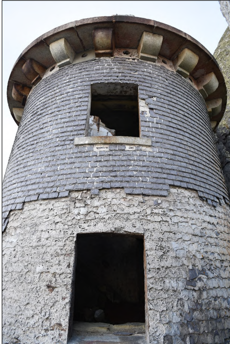
Photograph 29: Valentia Slate Cladding to Upper Lighthouse With Wicklow Granite Detailing to Sill and Upper Corbel Plinth.
