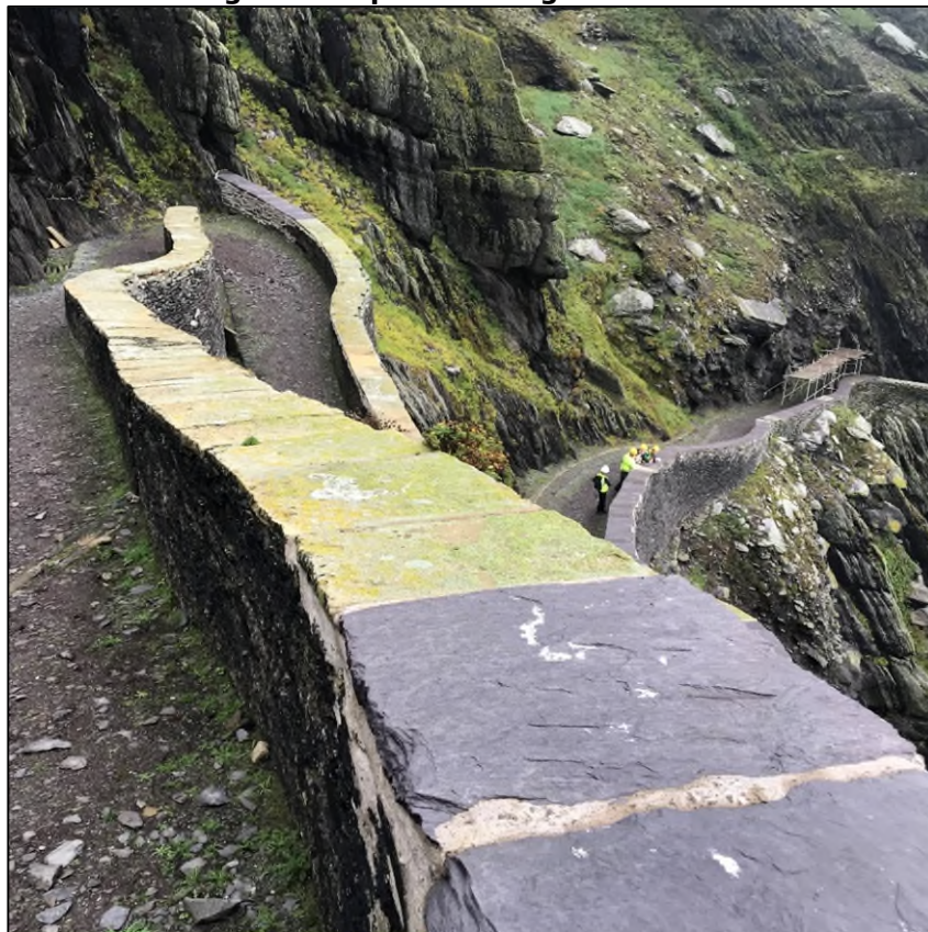
Photograph 14: Lighthouse Road Upper. Mix of Yorkshire Flagstone and "New" Valentia Slate Caps on Skellig Sandstone Rubble Wall.
