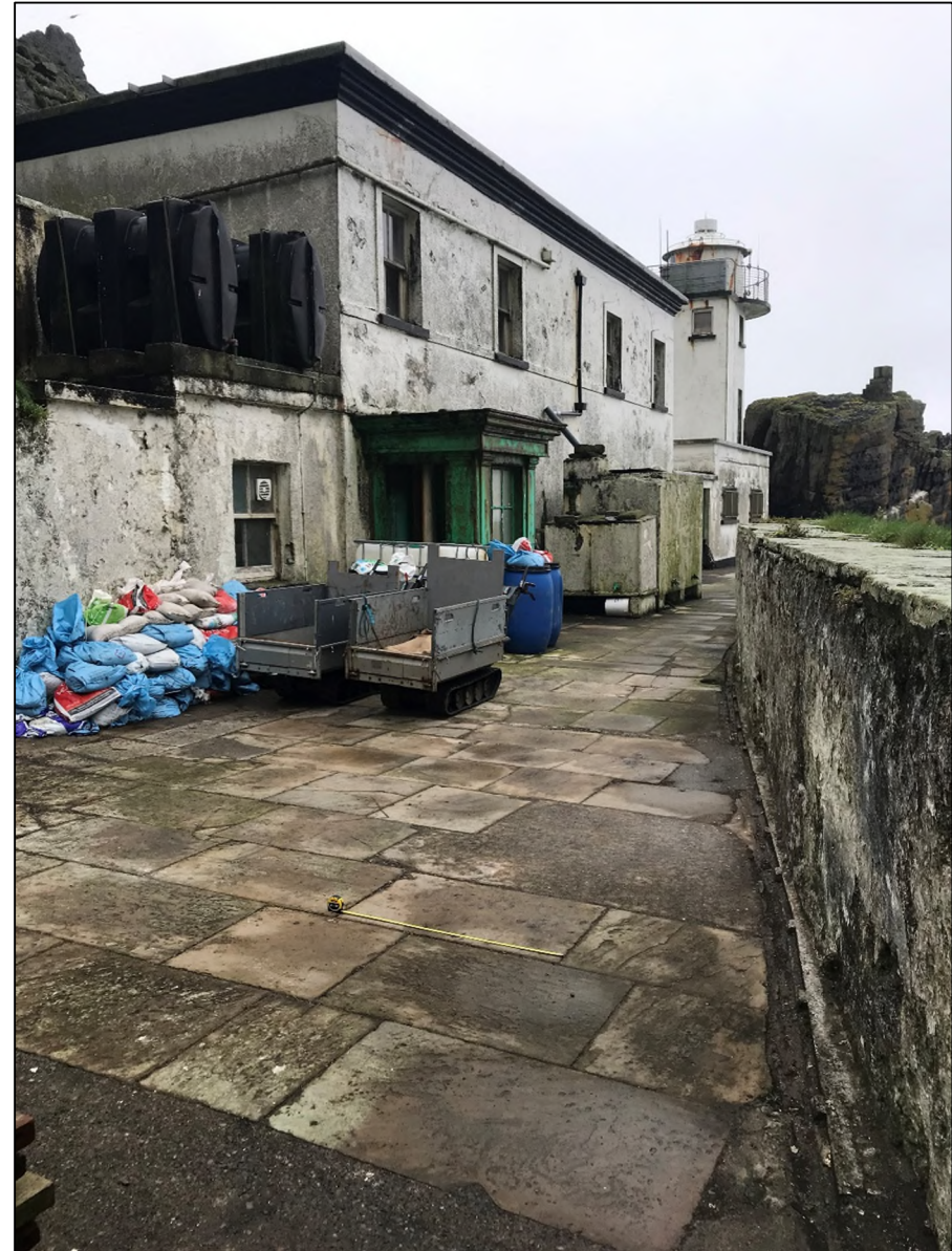
Photograph 2: Lower Lighthouse View to Southwest. Note Yorkshire Flagstones and Flagstone Caps to Safety Wall.
