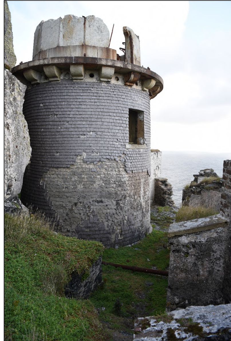
Photograph 30: Valentia Slate Cladding to Upper Lighthouse With Wicklow Granite Detailing to Sill and Upper Corbel Plinth.
