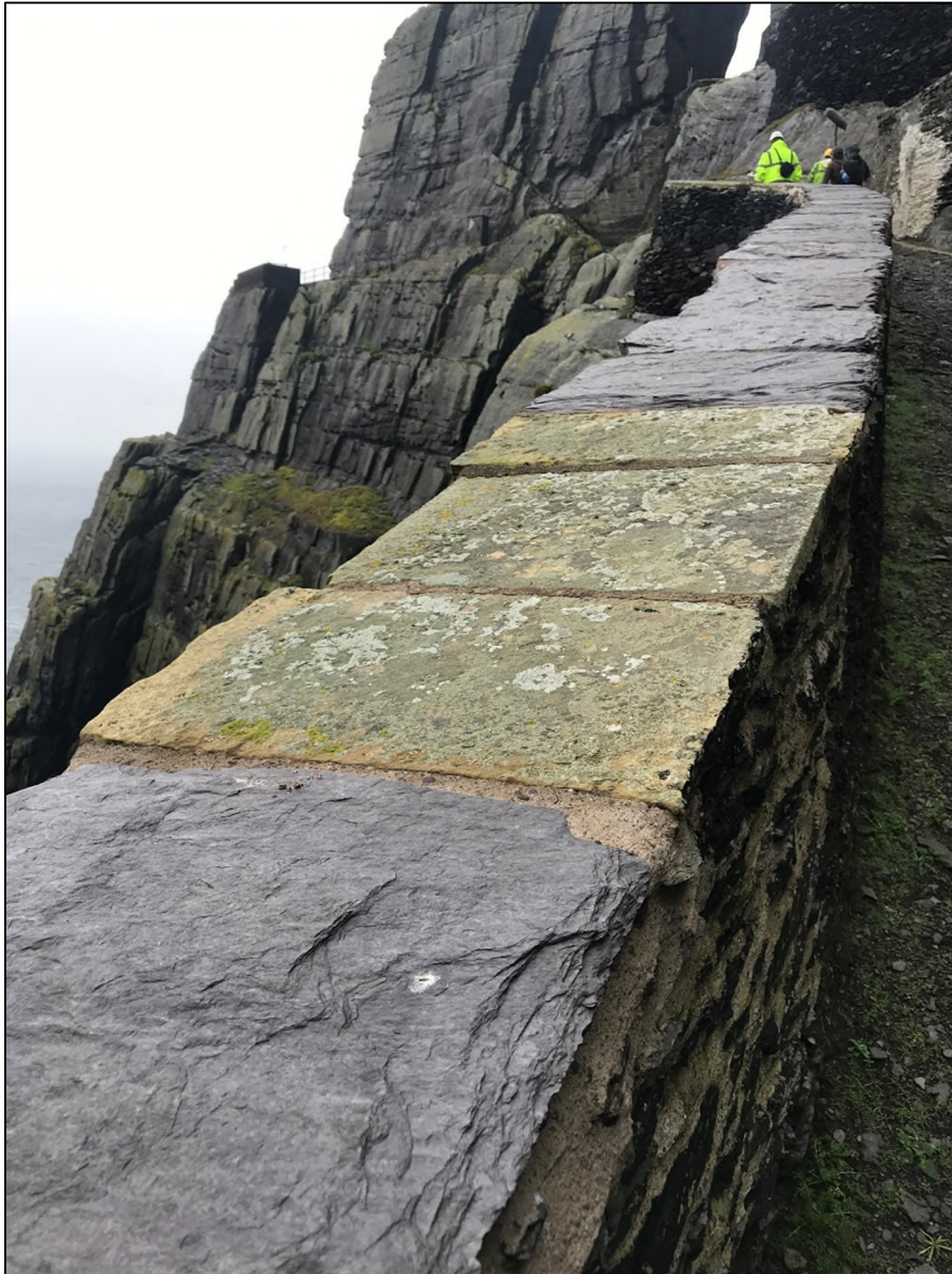
Photograph 11: Lighthouse Road Upper Section. Mix of "New" Valentia Slate and Yorkshire Flagstone Caps on Skellig Sandstone Rubble Wall.
