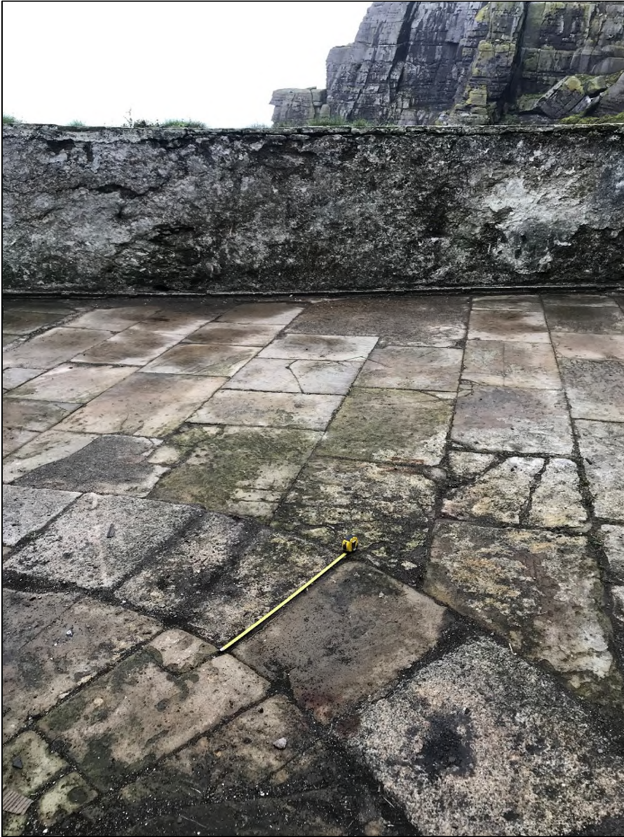
Photograph 5: Lower Lighthouse View to Northwest. Yorkshire Flagstones and Wicklow Granite Setts (curved with tape).
