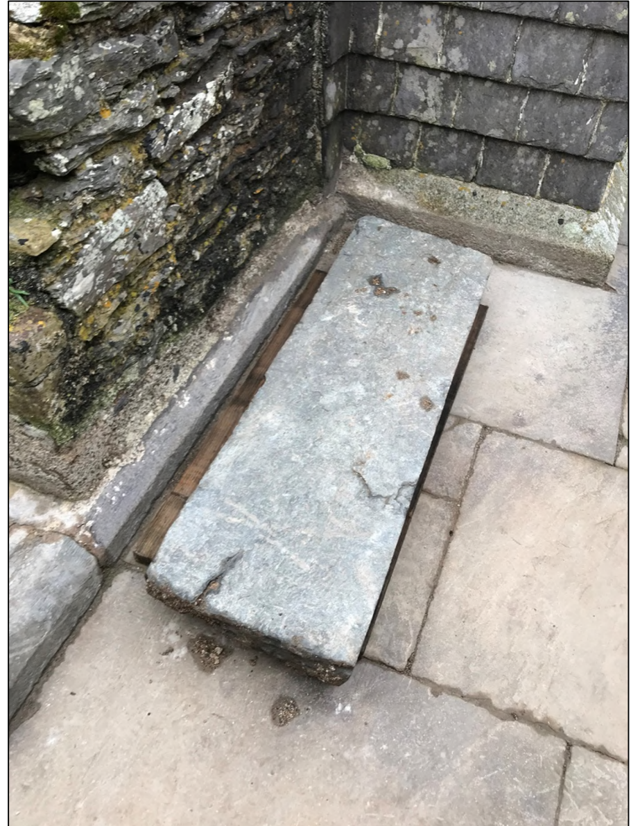
Photograph 20: Detail of Valentia Slate Base Plinth to Lighthouse Keepers' Cottages. Note Valentia Slate Plug.
