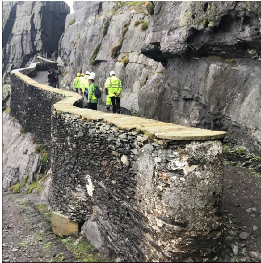
Photograph 13: Lighthouse Road Upper Section Dog-leg. Yorkshire Flagstone Caps on Skellig Sandstone Rubble Wall.
