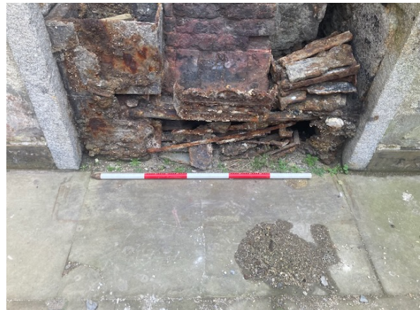
Fig. 19. House 2, kitchen, rust stain of iron fender.
