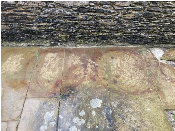
Fig. 18. Side yard, House 2, rust stains of barrels.
