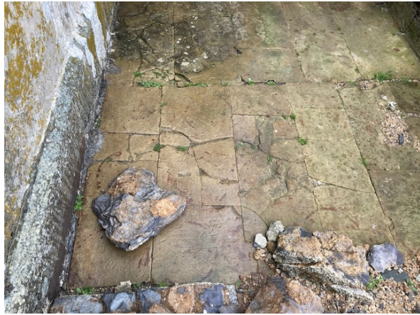
Fig. 17. Shed 21, centre room, cask rust marks.
