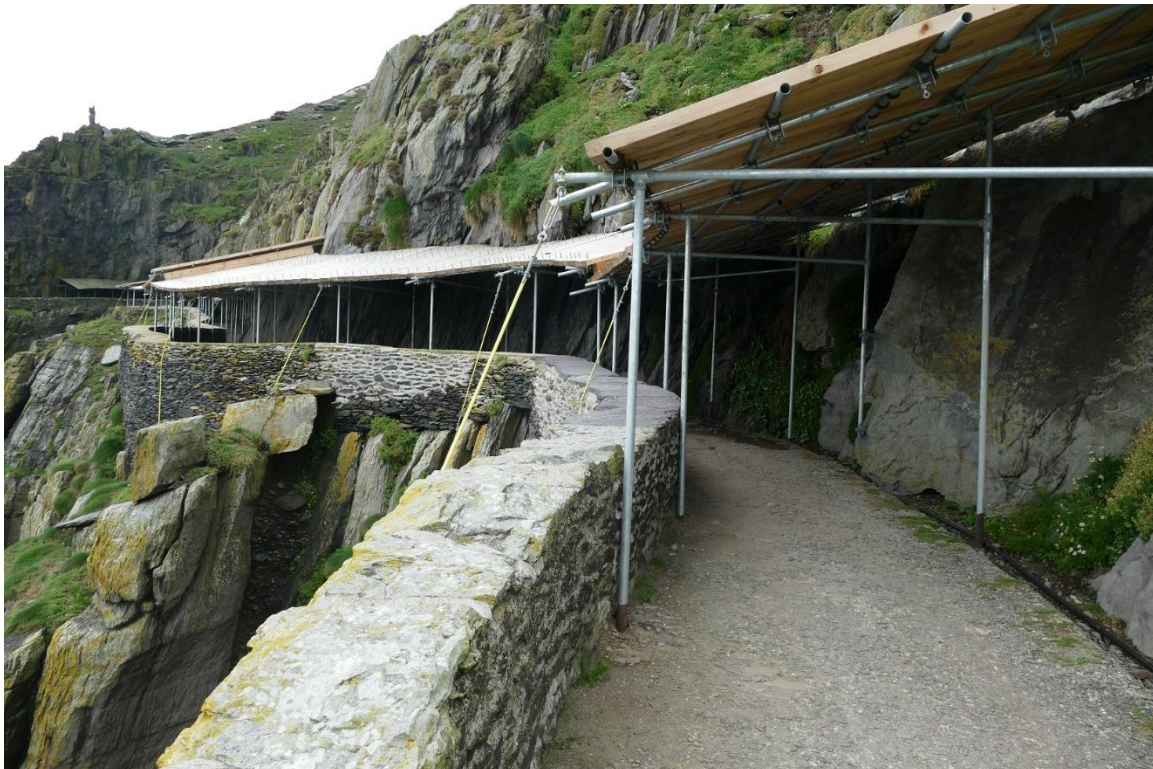
Fig. 38. - View of the canopy installed at the Lower Lighthouse road following the rock fall that occurred on 13 th June 2022
