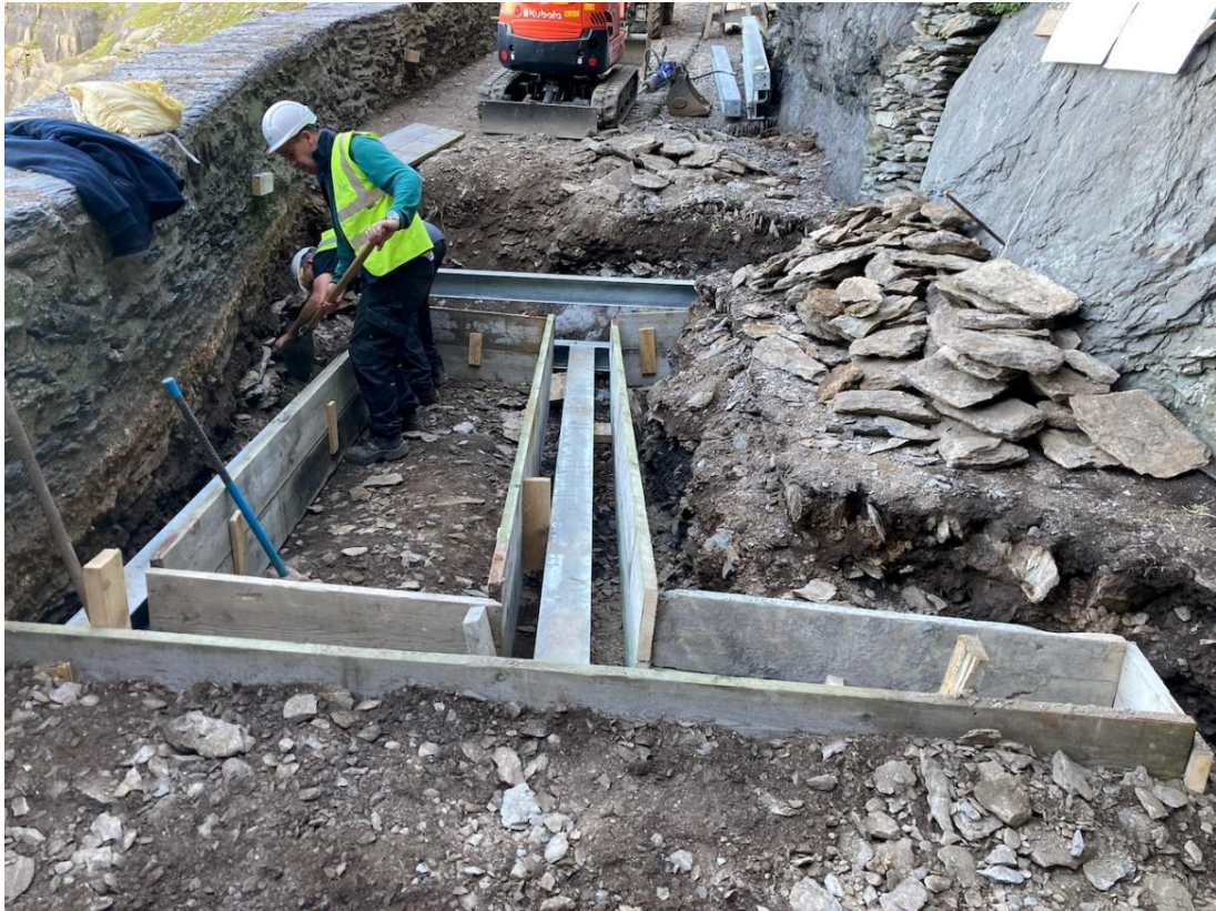
Fig. 46. - Crash Deck No. 3 – Installation of concrete foundation and associated ground works on site (Photo taken by Alan Hayden)
