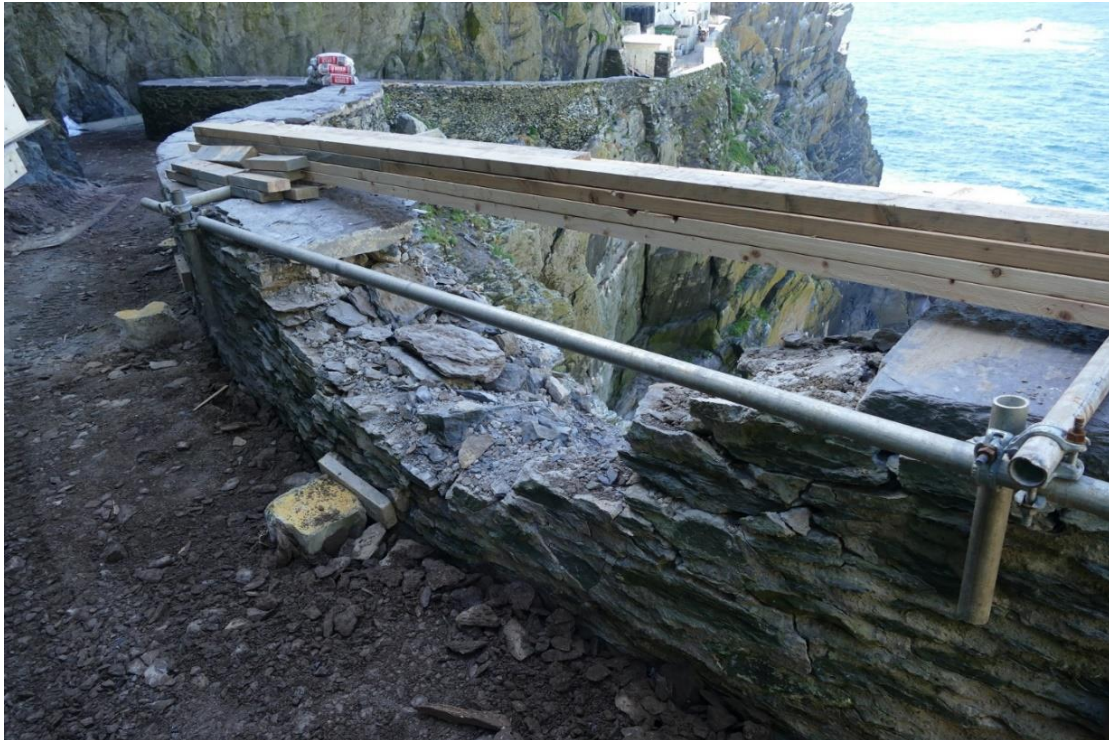
Fig. 41. - Temporary safety railing installed on site by OPW where the rock fall occurred in the location of crash deck no. 2 on the Upper Lighthouse road
