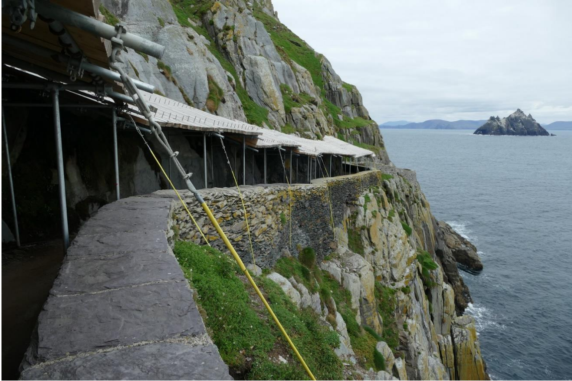
Fig. 37. - View of the canopy installed at the Lower Lighthouse road following the rock fall that occurred on 13 th June 2022
