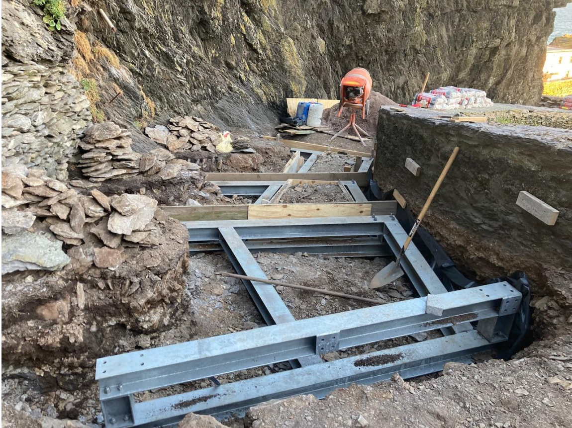
Fig. 48. - Crash Deck No. 3 – Installation of steel foundation on site (Photo taken by Alan Hayden)
