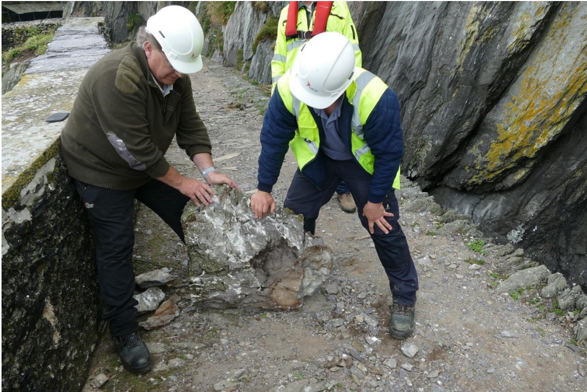
Fig. 33. - View of the existing rock from the rock fall that occurred on 13 th June 2022 on the Lower Lighthouse road
