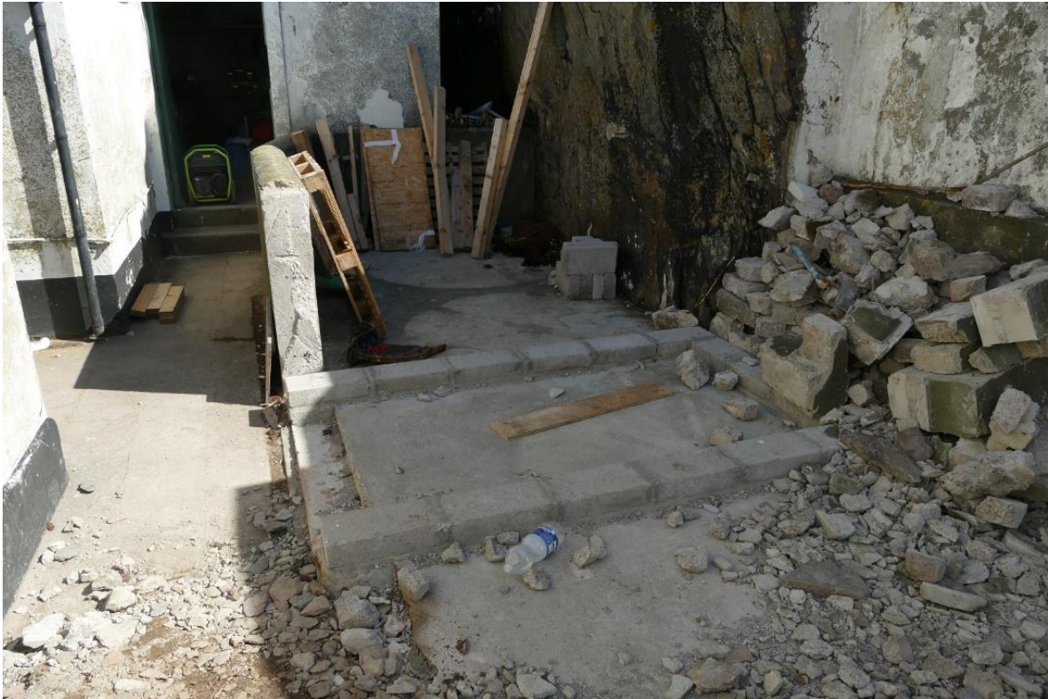
Fig. 16. - Foundation for the proposed composting toilet installed at the Lower Lighthouse compound
