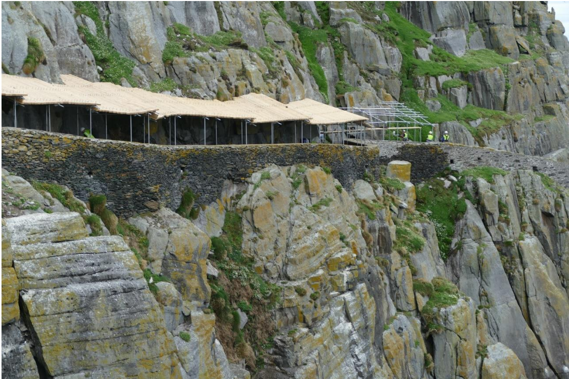
Fig. 35. - View of the canopy being installed at the Lower Lighthouse road following the rock fall that occurred on 13 th June 2022
