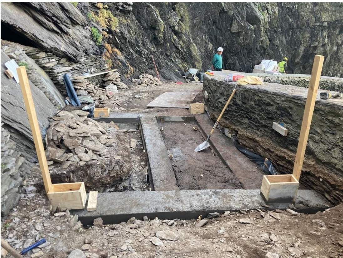
Fig. 47. - Crash Deck No. 3 – Installation of concrete foundation and associated ground works on site (Photo taken by Alan Hayden)
