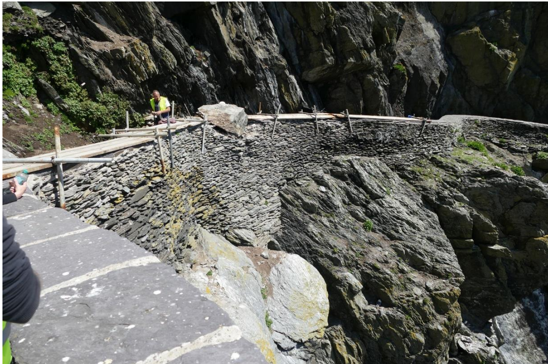
Fig. 40. - View of the rock fall in the location of crash deck no.2 on the Upper Lighthouse road
