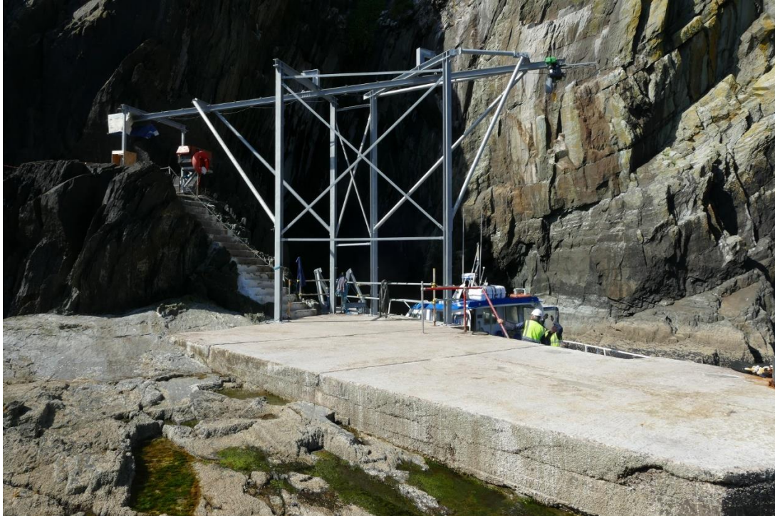
Fig .42. - Crane installed at the landing pier by Eamon Costello (Kerry) Ltd to facilitate lifting of steelwork and other heavy construction materials
