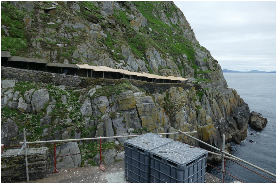
Fig. 34. - View of the canopy being installed at the Lower Lighthouse road following the rock fall that occurred on 13 th June 2022
