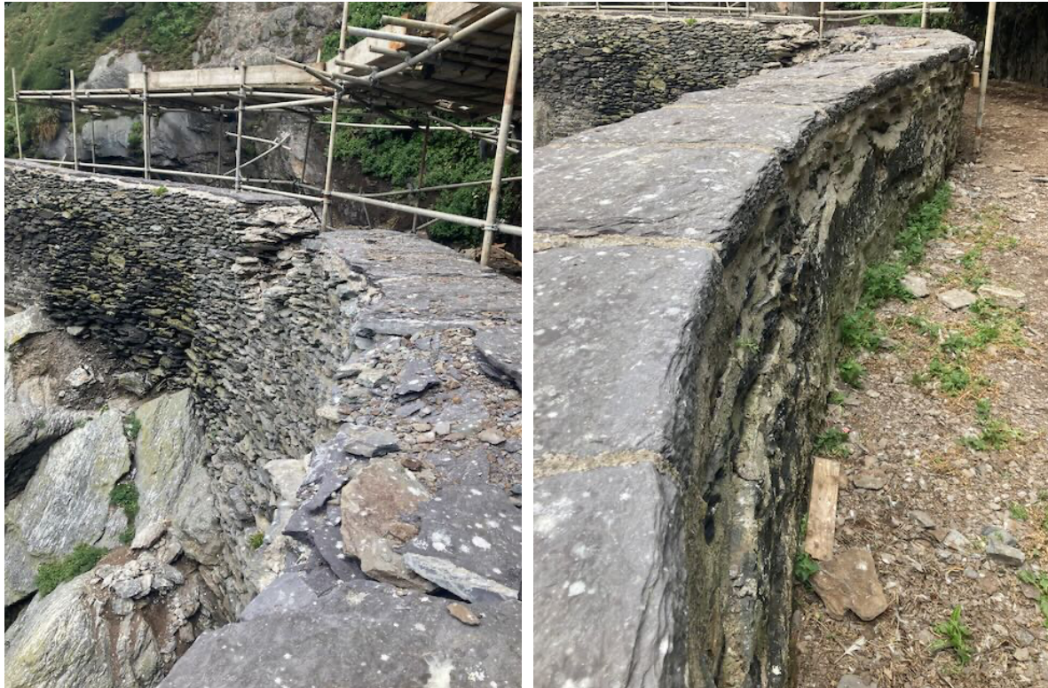
Photographs of the damaged section of the wall.
