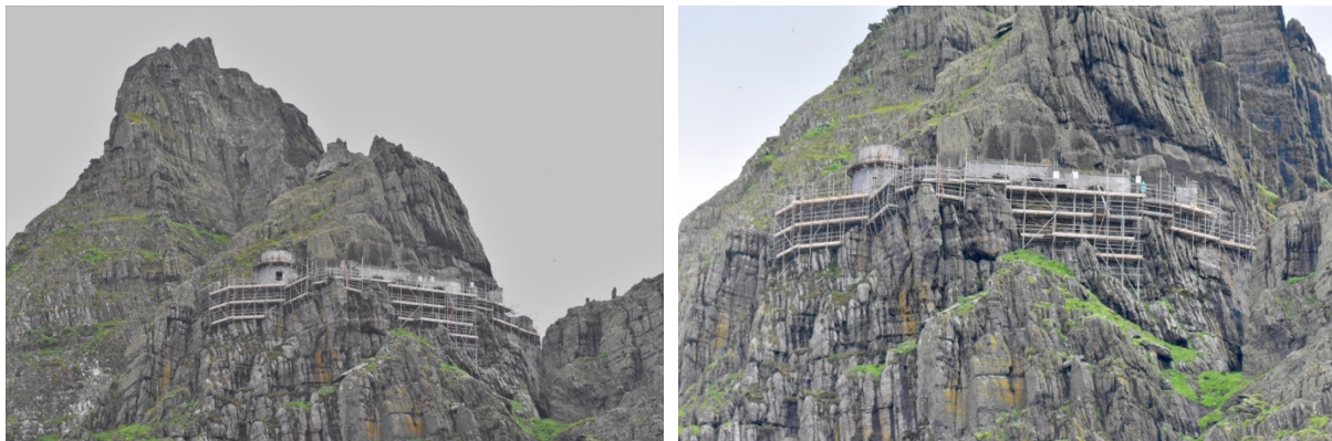
Fig. 3. The dramatic scaffolding erected by Brendan O'Connor and the OPW Skellig crew to facilitate the work on the wall (photographs by Brian Power).
