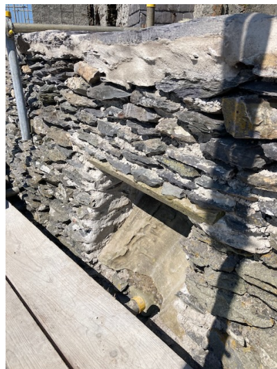
Fig. 6. Before & after photographs of parapet wall and details of rubbish chute behind House 1
