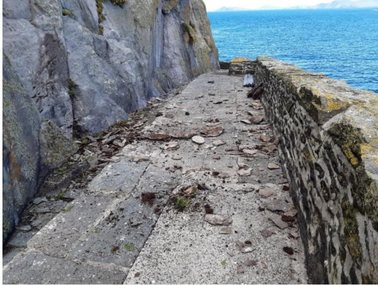
Figure 8 - Fallen debris from safety sweeps
