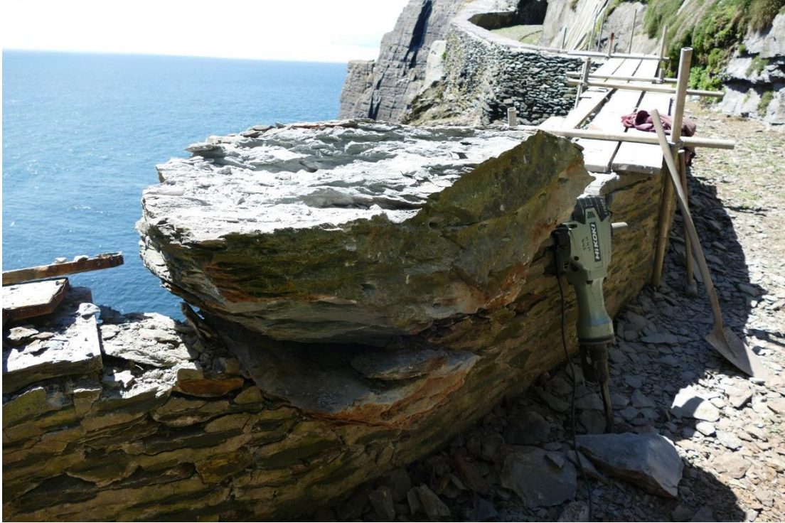
Figure 12 - Example of rock fall on the Upper Lighthouse Road in the 2022 season
