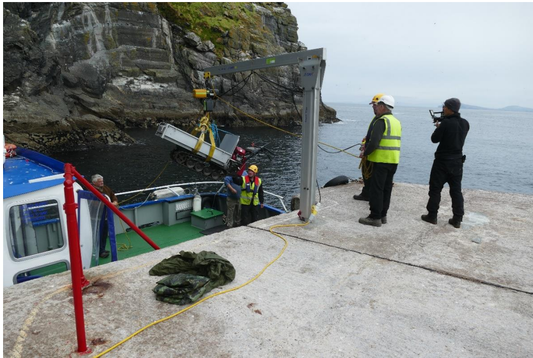
Figure 32 - View of the demountable hoist at the landing pier
