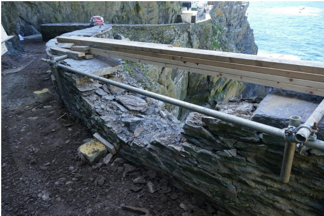
Figure 13 – Example of temporary safety railing installed at the Upper Lighthouse Road by OPW in the 2022 season
