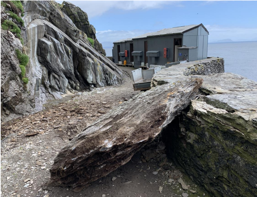
Figure 32 - Rock Fall on 27th July 2020
