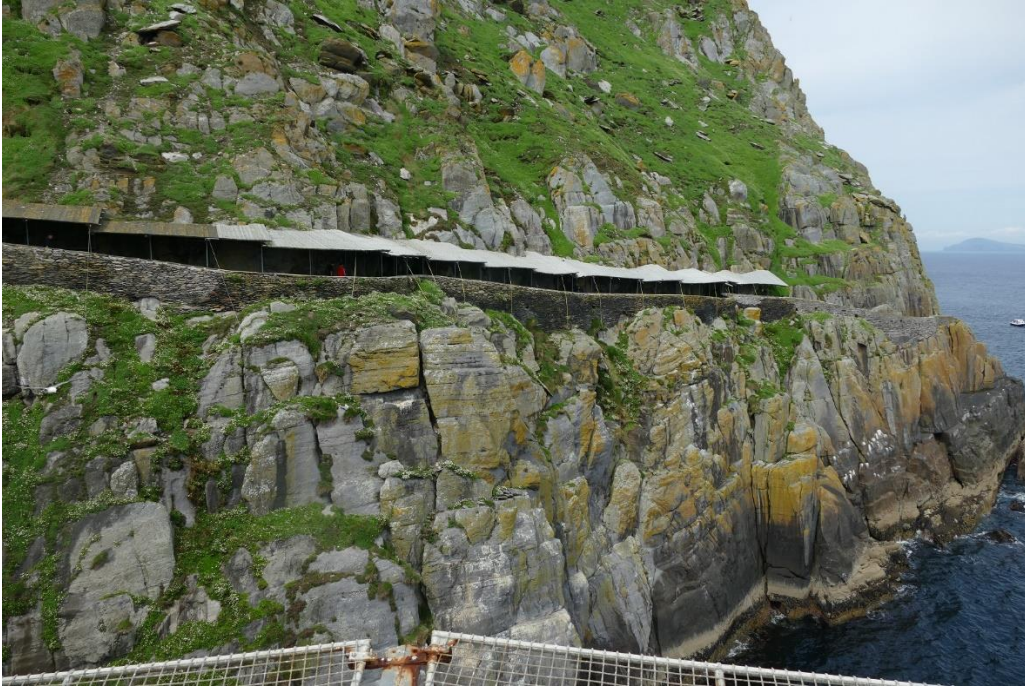
Figure 35 - View of the canopy installed at the Lower Lighthouse road following the rock fall that occurred on 13th June 2022
