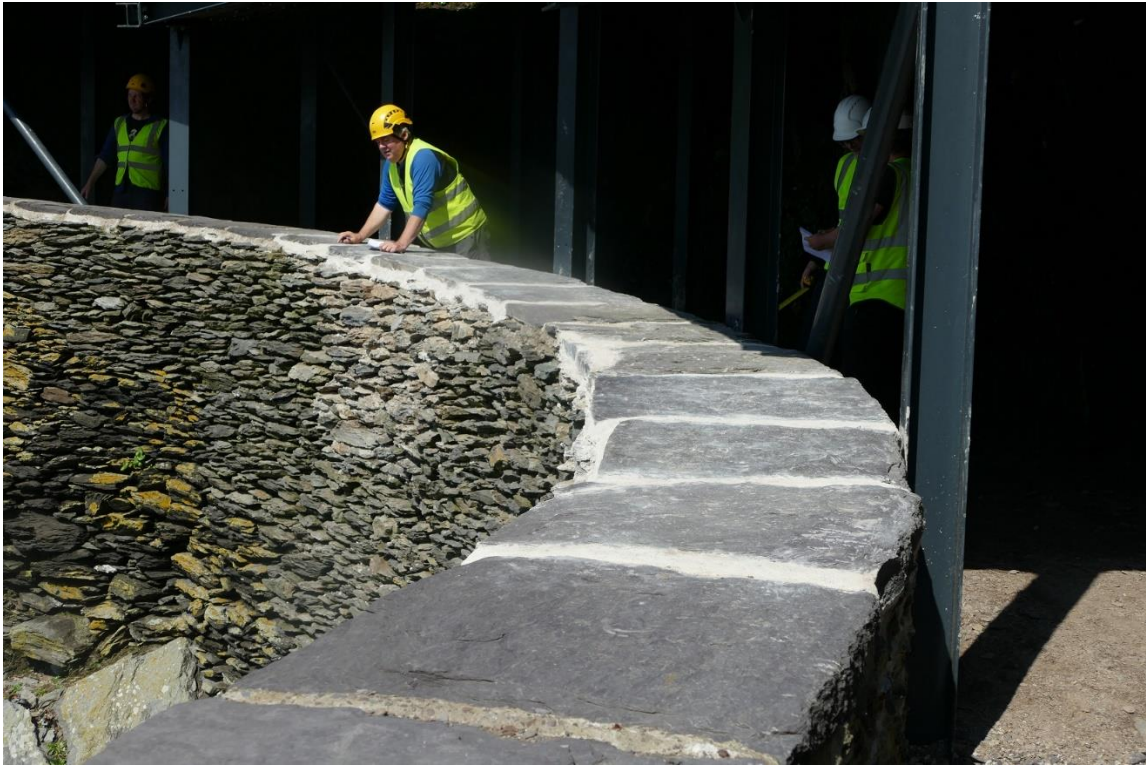
Figure 9 - Completed repair works to the damaged section of sea wall on the Upper Lighthouse Road
