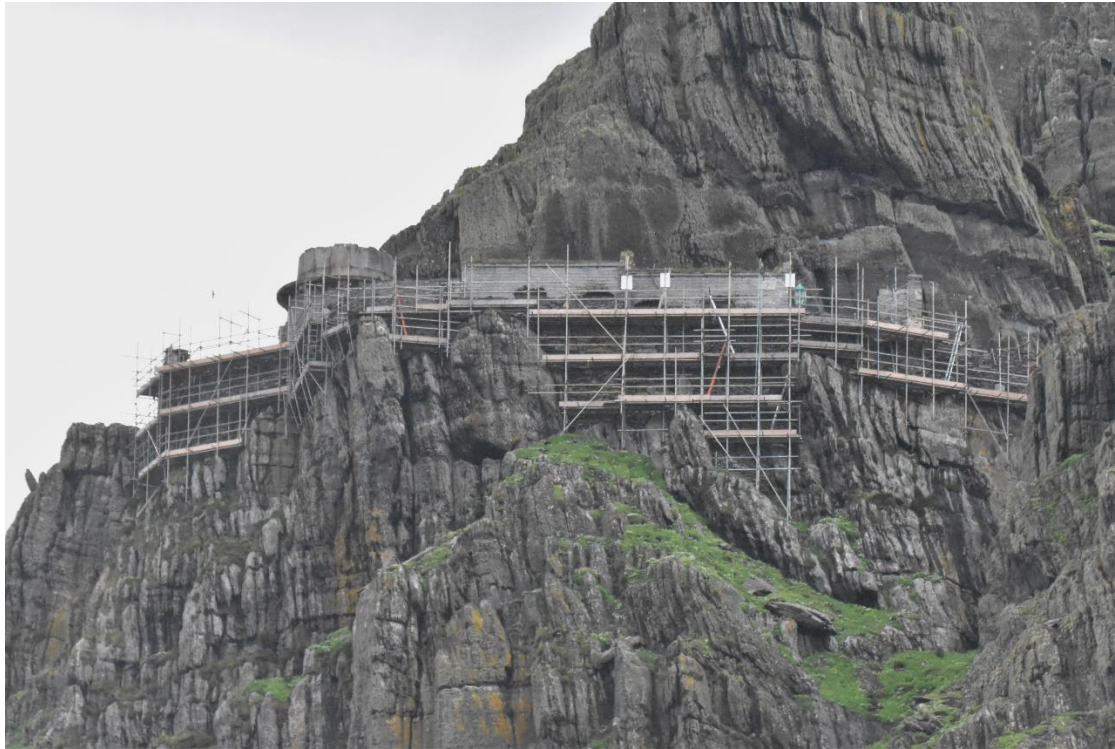
Figure 17 - View of the scaffolding installed at the Upper Lighthouse on Sceilg Mhichíl
