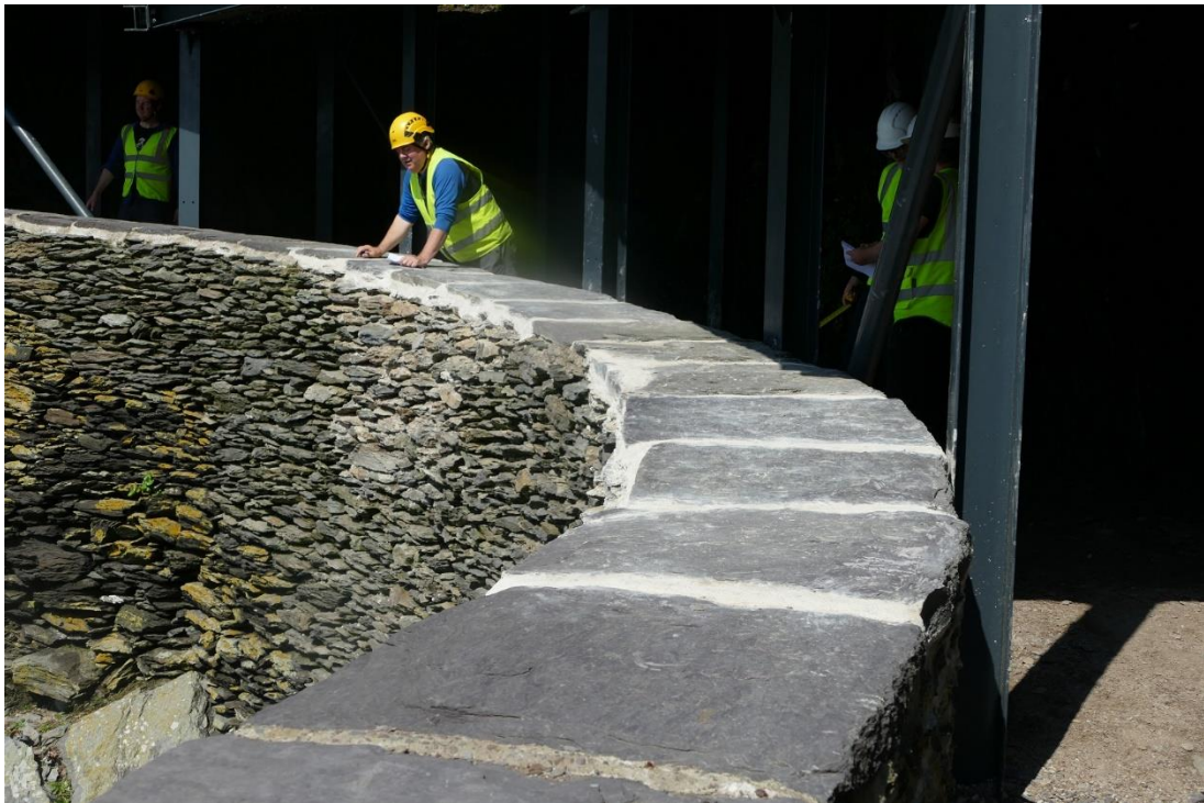
Figure 38 - Damaged of section of sea wall repaired by OPW in the 2023 season
