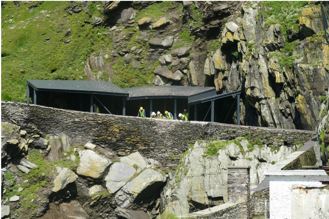
Figure 10 - Completed repair works to the damaged section of sea wall on the Upper Lighthouse Road
