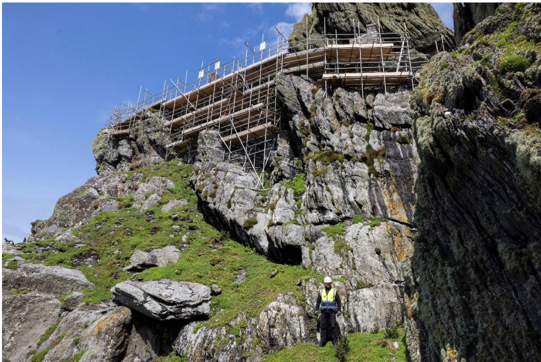
Figure 16 - View of the scaffolding installed at the Upper Lighthouse on Sceilg Mhichíl © Photographic Archive, National Monuments Service, Government of Ireland
