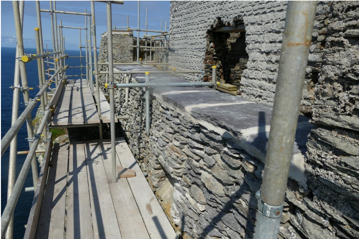
Figure 19 - Repair works carried out by OPW to the sea wall at the Upper Lighthouse
