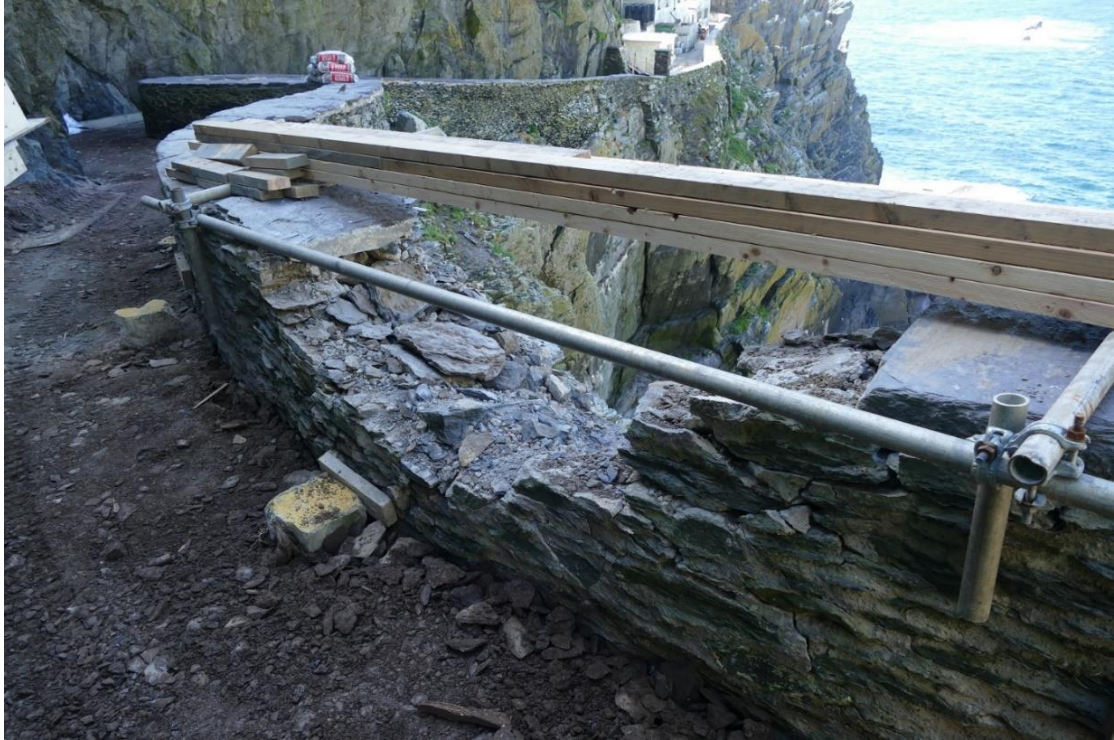
Figure 34 - Temporary safety railing installed on site by OPW where the rock fall occurred in the location of crash deck no. 2 on the Upper Lighthouse road
