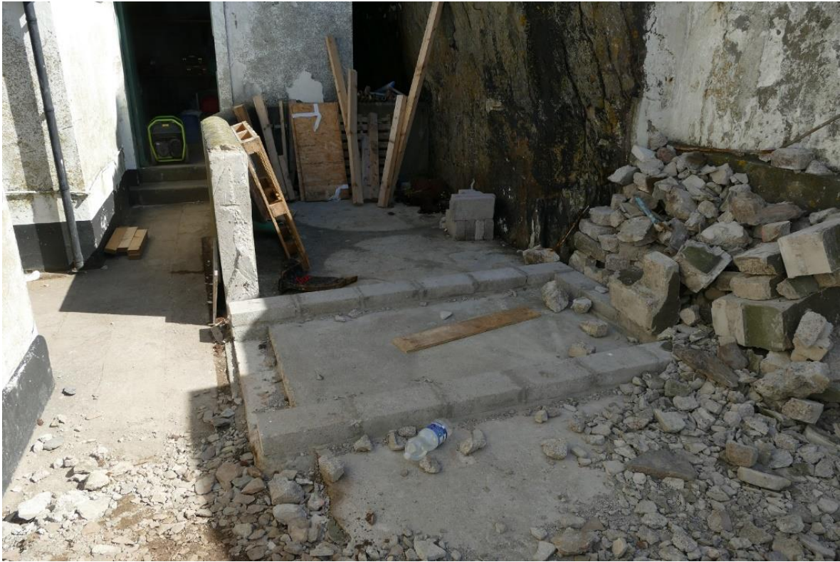
Figure 13 - Foundation for the proposed composting toilet installed at the Lower Lighthouse compound
