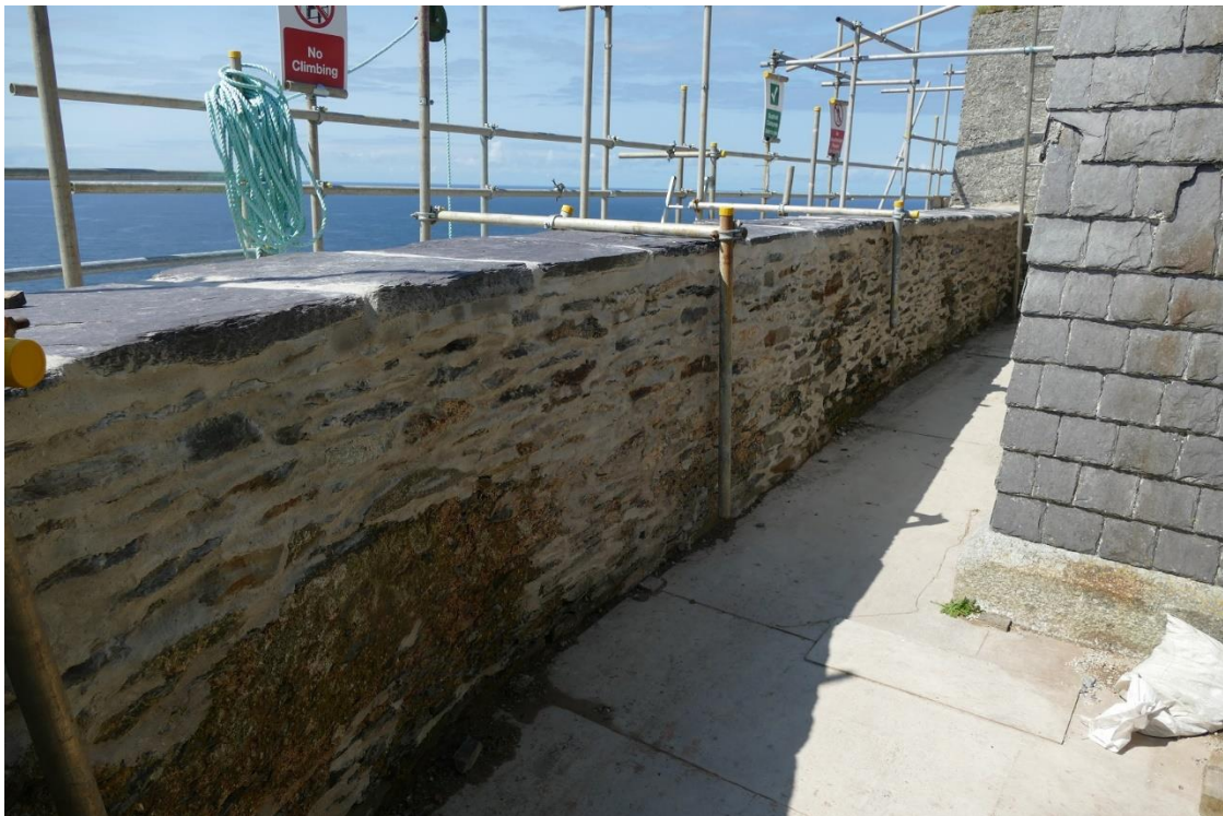
Figure 18 - Repair works carried out by OPW to the sea wall at the Upper Lighthouse
