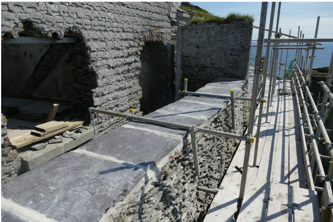
Figure 20 - Repair works carried out by OPW to the sea wall at the Upper Lighthouse
