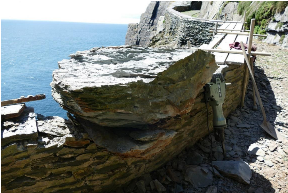
Figure 33 - View of the rock fall in the location of crash deck no.2 on the Upper Lighthouse road
