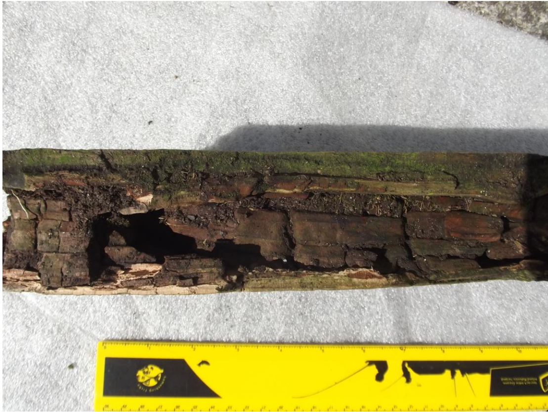
Figure 3. Severe decay in core of board, with relatively intact surface layer.
