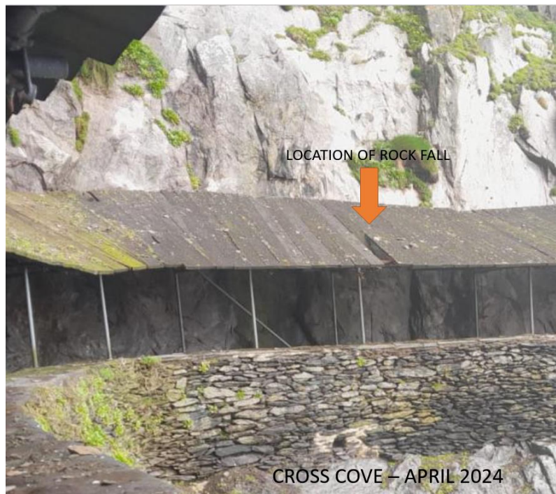
Image: Cross Cove Crash Deck – Location of board damaged by rockfall.
