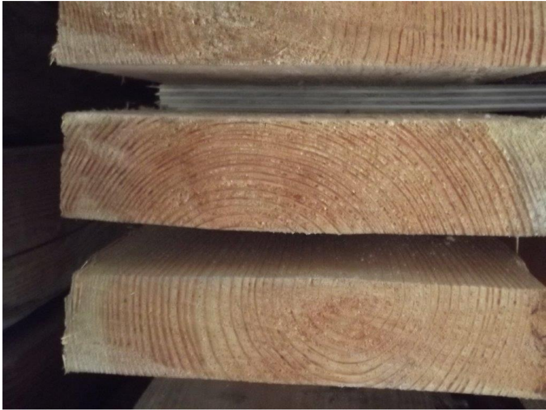
End-grain of slow-grown material. Stain to sapwood at edge of two lower boards.
