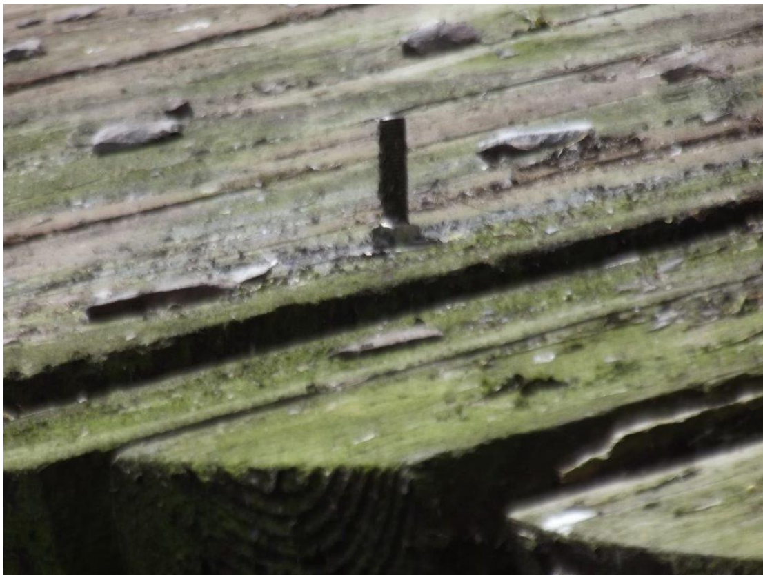
Figure 2. J bolt through boards. Note loose stones from above.
