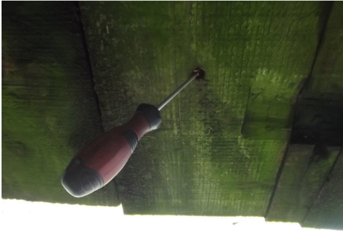
Figure 4. Decay at hole with screwdriver inserted deeply.
