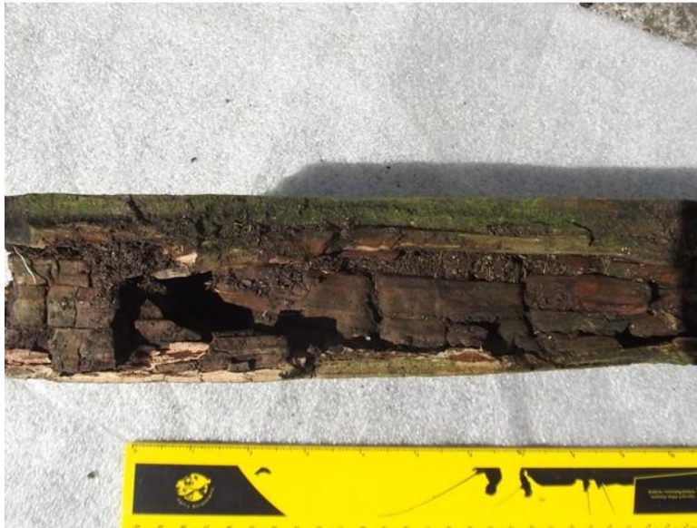
Image: Photo of board sample from Report 002413 - severe decay in core
