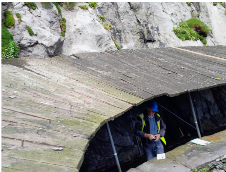
OPW Images: General Views - Phase 1 of Cross Cove Crash Deck as of May 25 th 2024
